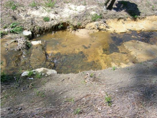
Erosion Area, Cross Section #3 (SREV 6+65)
