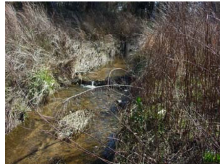
Photo 4: New central bar formation problem area (Station No. 18+65; view upstream; 2-20-2008).
