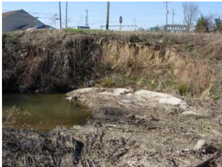
Photo 3: Severe bank failure, aggradation, and bar formation just downstream of culvert at head of restoration reach on (Station No. 10+05; view of left bank facing upstream; 2-20-2008).
