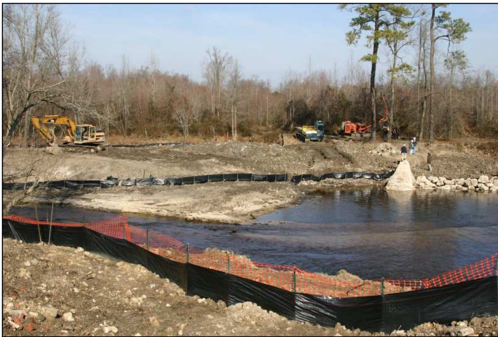
Photo 4. Debris disposal areas viewed from south bank—note remaining section of dam (January 2006)
