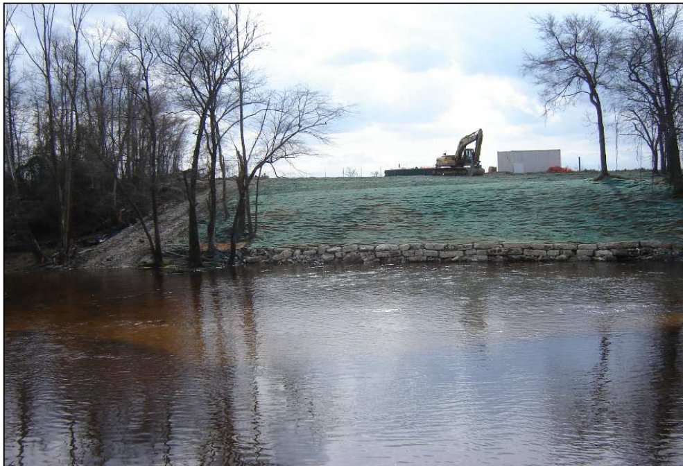
Photo 5. Concrete spillway debris placed as toe protection along re-graded south bank—note hydro-seeding (January 2006)
