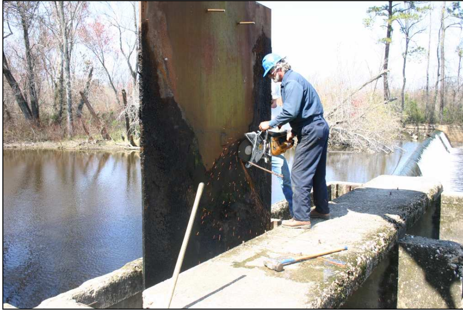
Photo 2. Removal of steel plate restricting water passage through the mill works foundation (March 2004)
