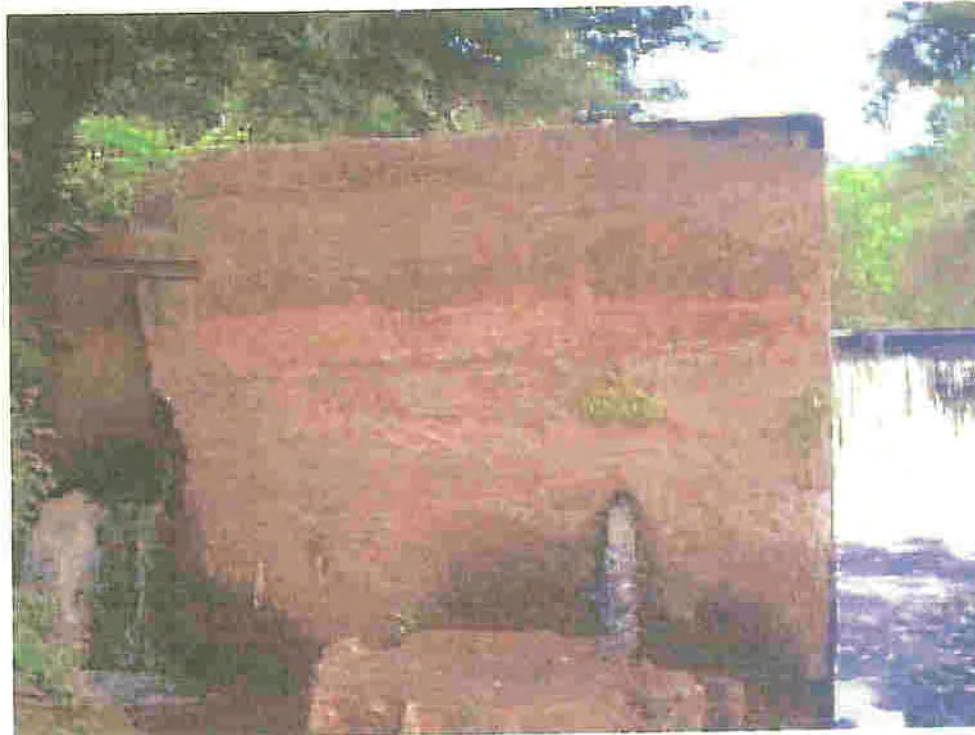
Photo 4: Downstream Leakage of Mill Foundation
