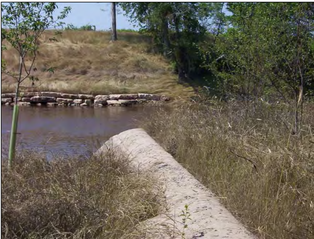
Photo 18. River Observation Point 9. Photo taken from the remnant dam structure (north bank) looking south at the toe protection placed at the location of the dam's south abutment and mill works. Little River, Johnston County.
