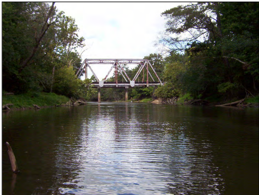
Looking upstream at the US 301 and railroad bridges following dewatering—note lower water surface elevation and stable, vegetated stream banks
