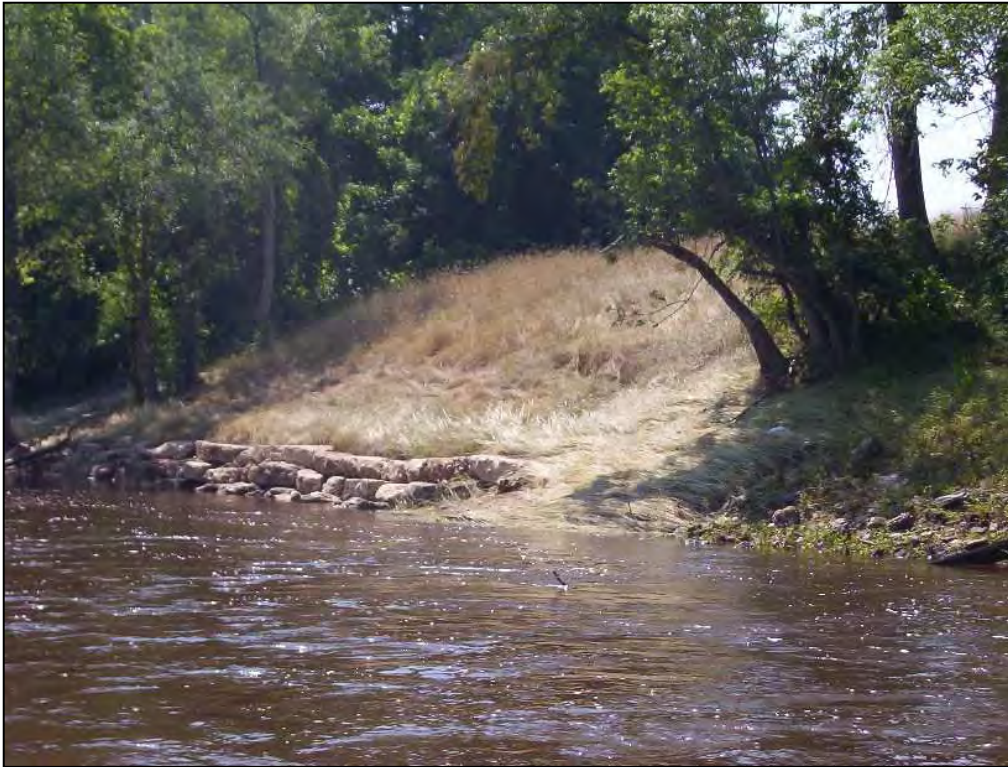
Photo 17. River Observation Point 9. Toe of slope protection along the south embankment, location of the dam's south abutment and mill works. Little River, Johnston County.
