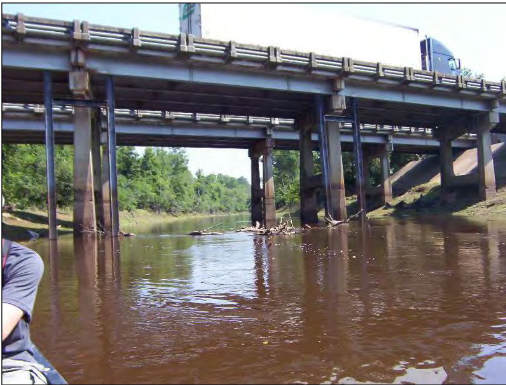
Photo 12. River Observation Point 7. Photo looking upstream at the I-95 overpass. Note: No evidence of scouring and only a small amount of debris among the pilings. Little River, Johnston County.
