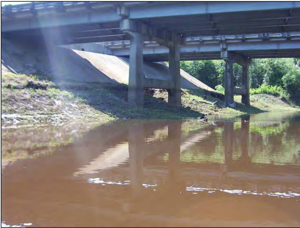
Photo 11. River Observation Point 7. Well established herbaceous vegetation along the north banks of the river at the I-95 overpass. Note the vegetation in the NCDOT right-of-way has been mowed. Little River, Johnston County.
