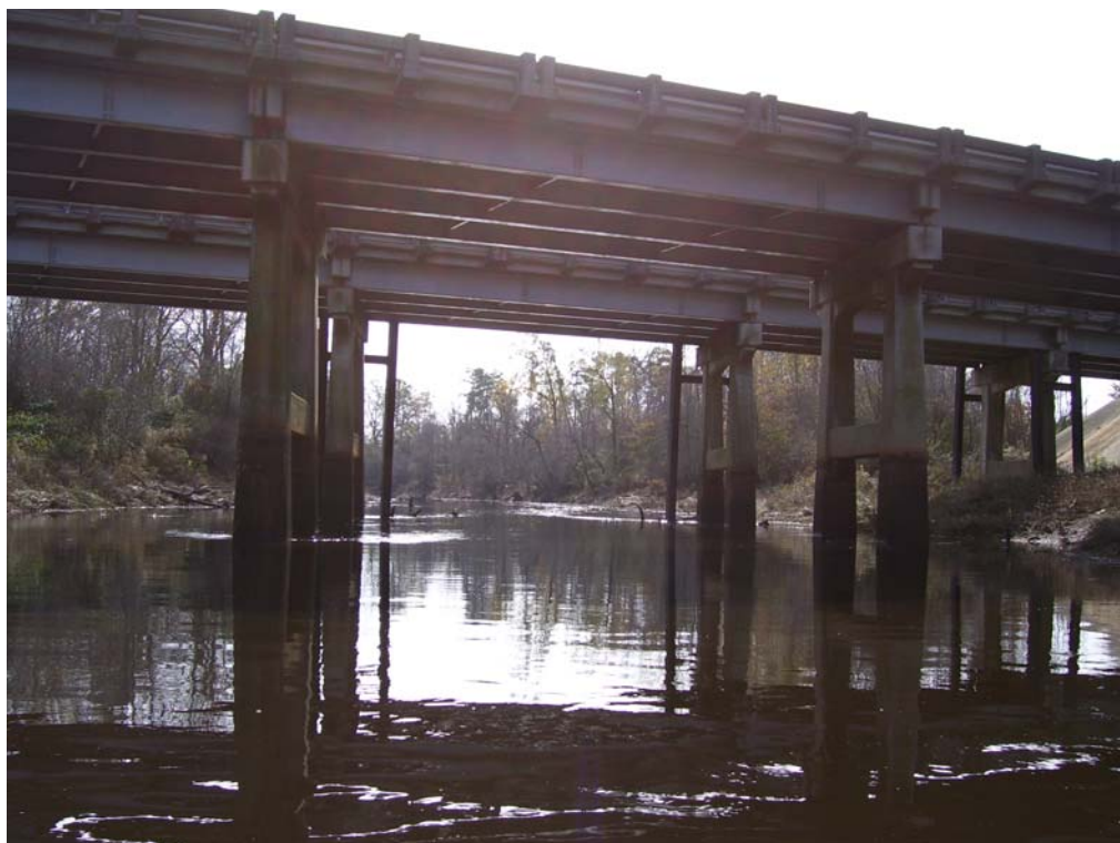
Photo 4. River Observation Point 7. The bridge pilings (I-95) located within the Little River contained only a small amount of debris and no evidence of scouring was observed. Little River, Johnston County.
