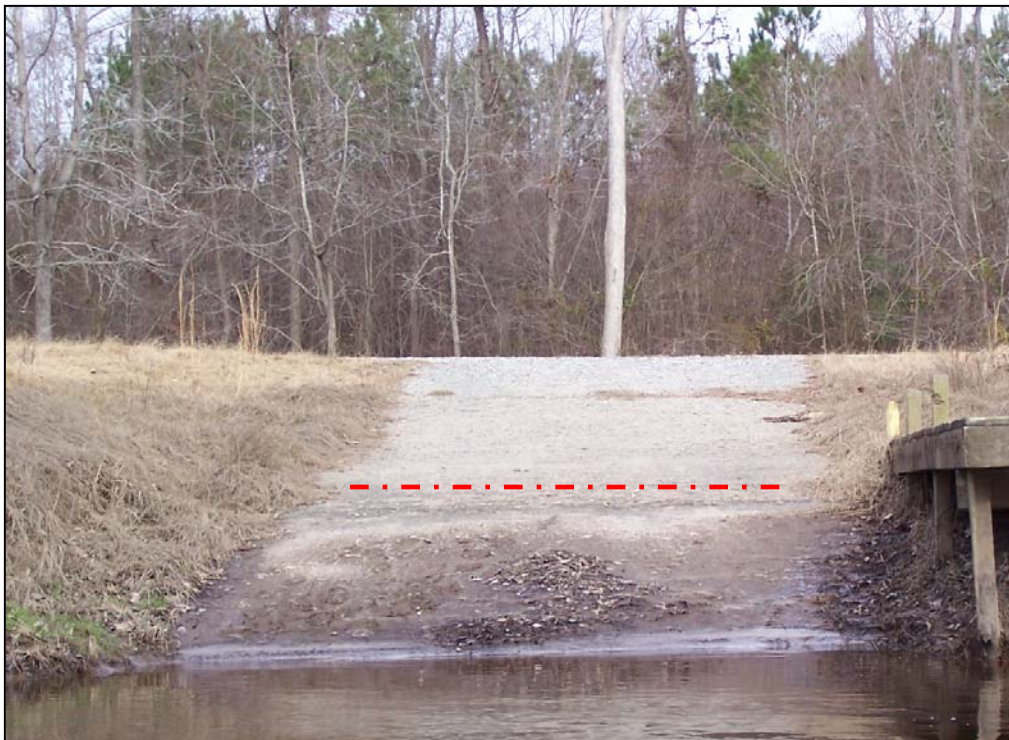
Photo 2. River Observation Point 2: Sediment deposition and high water mark (red line) at the Wildlife Resource Commission boat ramp. Little River, Johnston County.
