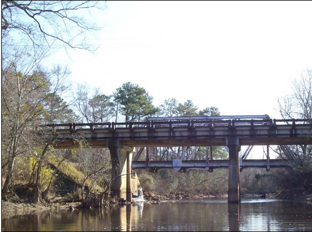
Photo 15. River Observation Point 13: The bridge pilings (US 301) located within the Little River contained no woody debris and no evidence of scouring was observed. Little River, Johnston County.
