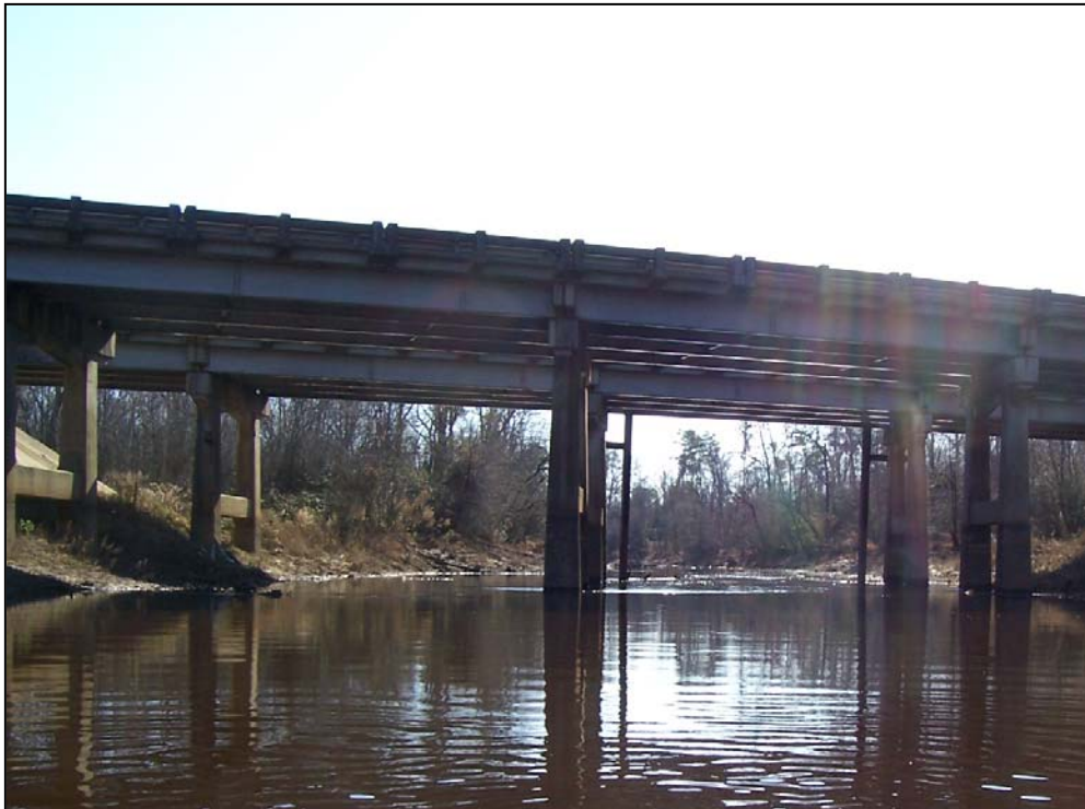
Photo 5. River Observation Point 7: The bridge pilings (I-95) located within the Little River contained no woody debris and no evidence of scouring was observed. Little River, Johnston County.
