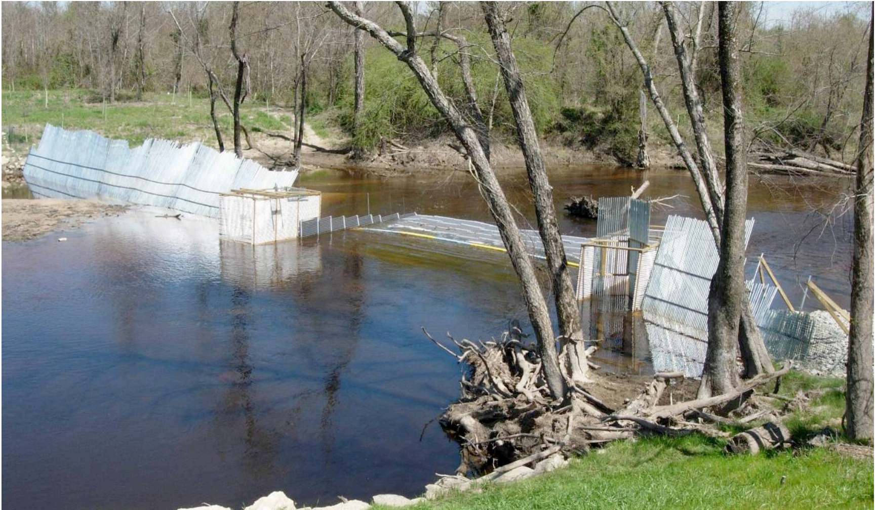
Figure 3. Installed fish weir on the Little River, with resistance board weir in center and picket weir sections on both sides of live cages. Picture taken on March 30, 2007, view is looking downstream.
