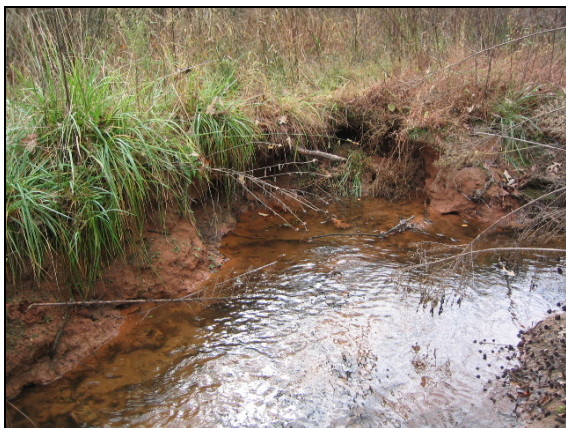
Issue Photo 3 and 4 – Station 16+90 Bank failure due to overland flow.
