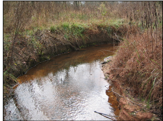
Issue Photo 2 – Station 11+00 Bank undercutting due to lack of vegetation.
