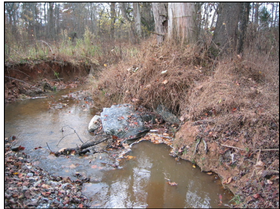
Issue Photo 9 – Station 13+40 Scour around upstream side of cross vane wing.
