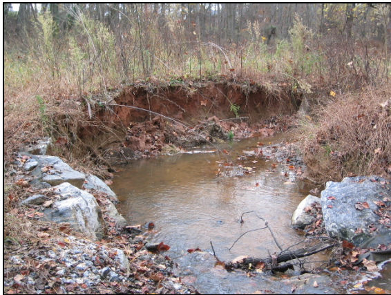
Issue Photo 8 – Station 13+70 Severe bank erosion.
