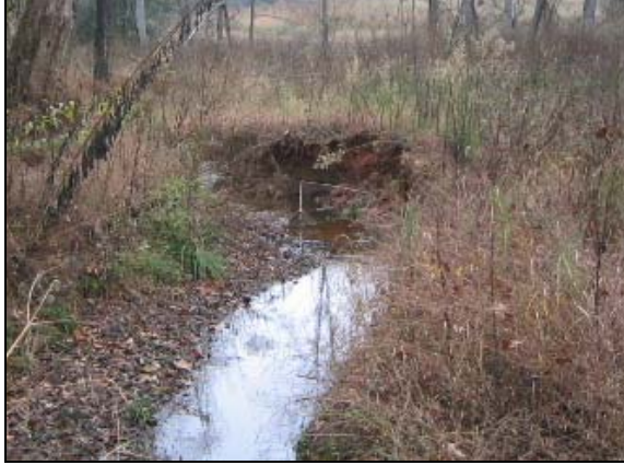
Issue Photo 6 – Station 15+80 Bank erosion due to lack of vegetation.
