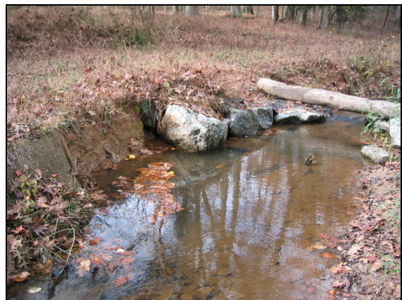
Issue Photo 9B – Station 19+70 Scour below cross vane.
