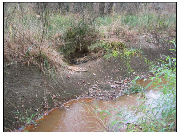
Issue Photo 5 – Station 10+40 Bank failure under matting.
