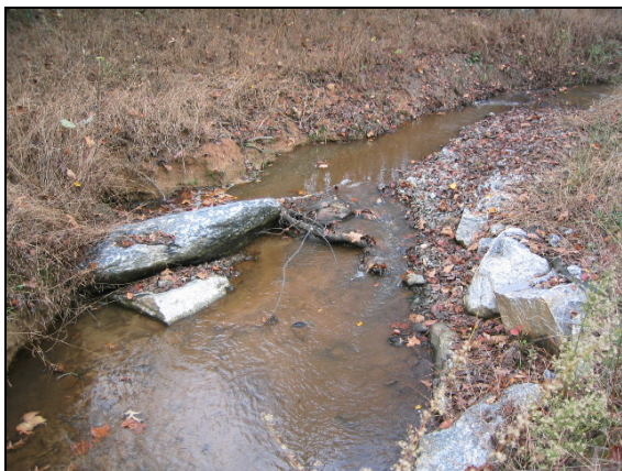
Issue Photo 9A – Station 18+50 Scour around upstream side of cross vane wing.
