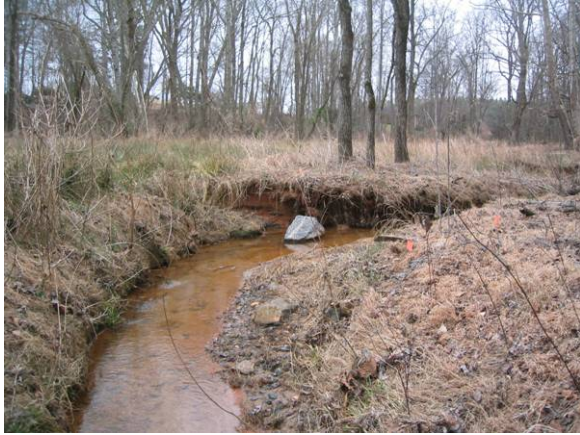
Issue Photo 3 Bank Erosion Outside Meander Bend Left Bank
