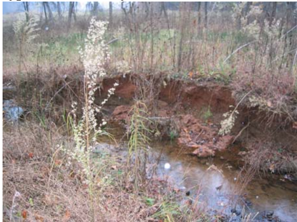
Issue Photo 1 Lyle Creek Pool near station 9+40. Typical Bank Slump on Left Bank
