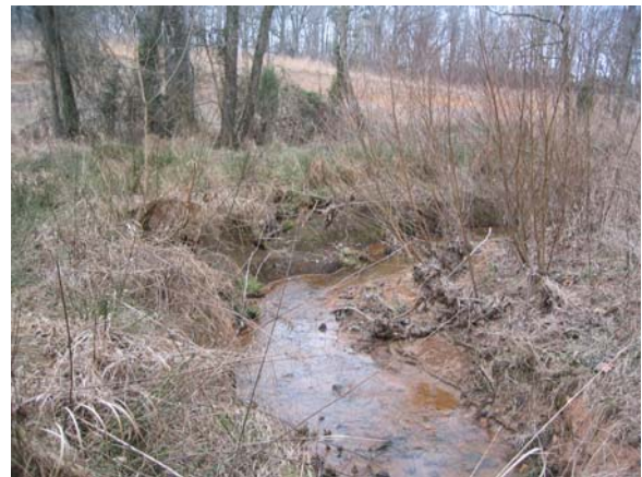
Lyle Creek Pool near station 11+90. Typical Bank Failure on Left Bank
