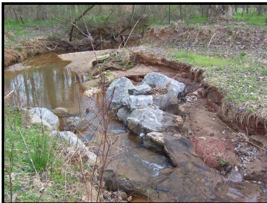
Figure 4—Typical Failing Structure
