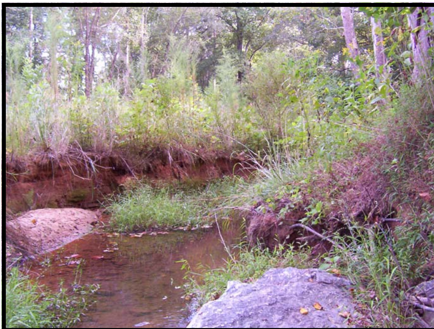
Figure 2—Typical Bank Scour
