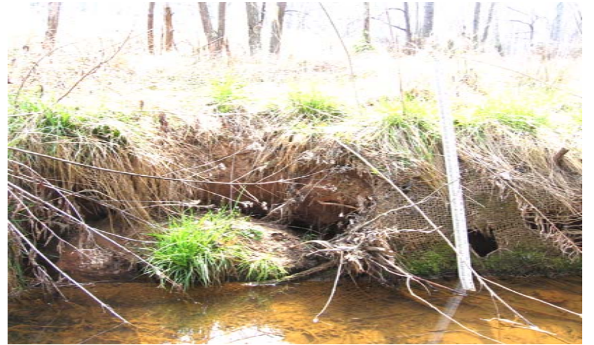
4. Bank Erosion: Severe-3/30/06
