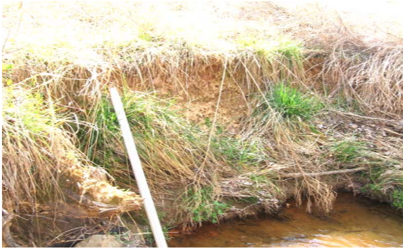
3. Bank Erosion: Moderate-3/30/06
