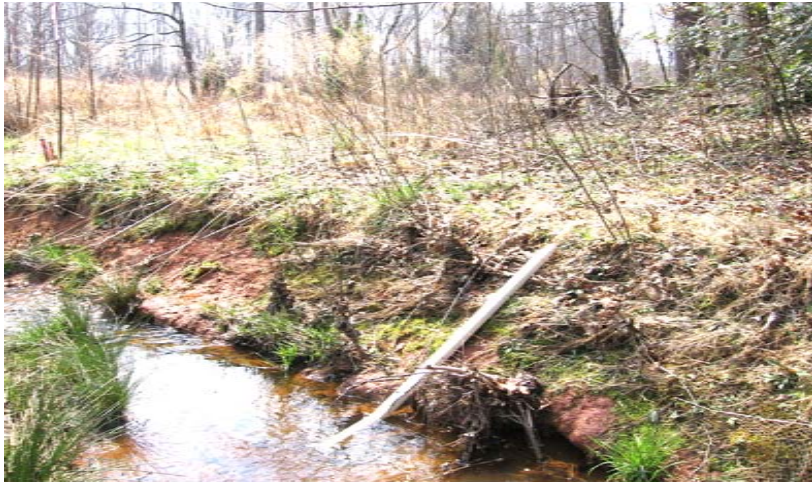
1. Bank Erosion: Moderate-3/30/06
