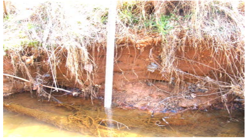
2. Bank Erosion: Severe-3/30/06
