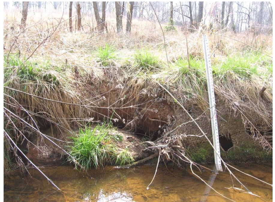
2. Bank Erosion: Severe-3/30/06
