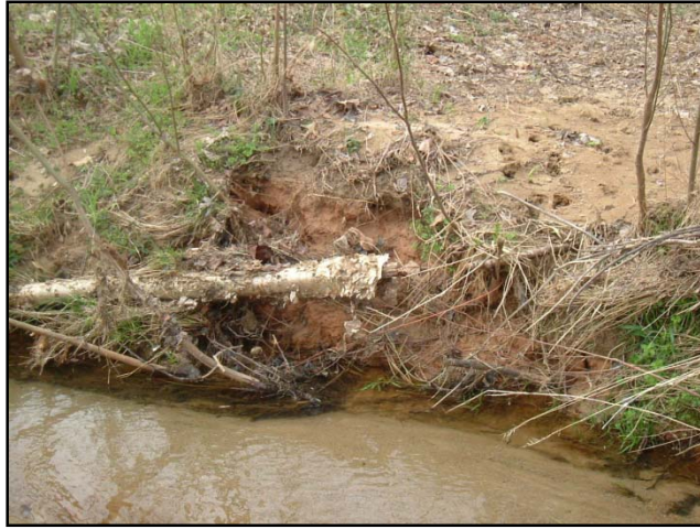
1. Moderate Bank Erosion-3/22/2007
