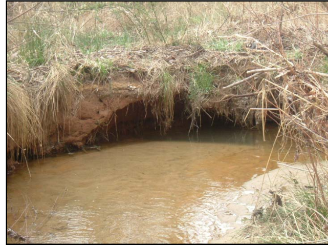
2. Severe Bank Erosion-3/22/2007
