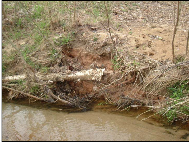
1. Moderate Bank Erosion-3/22/2007
