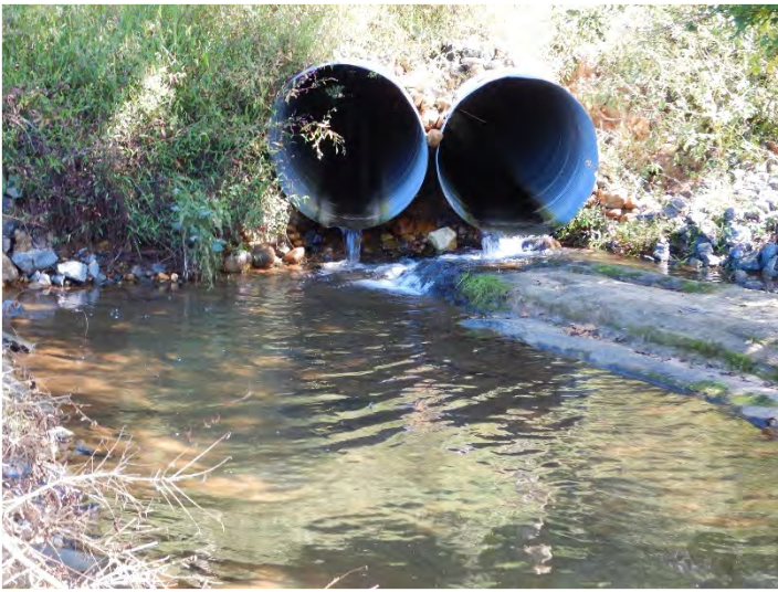
Hanks Branch R3 – Perched Culvert Outlet (9/27/2021)
