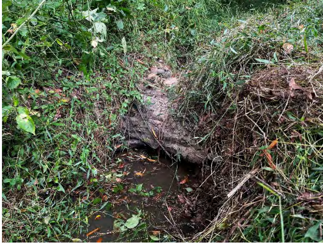
UT4 Reach 2, station 604+40 – Log sill piping (10/1/2023)
