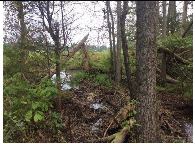
Initial Dam Breach near WC, Spoil, Debris – Looking Upstream (9/25/2018)
