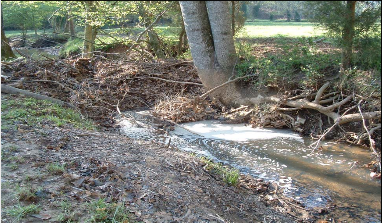
Photograph 11 – Looking downstream at debris jam across UTBC channel, right bank undercut with exposed roots upstream of jam (Station ~15+50).
