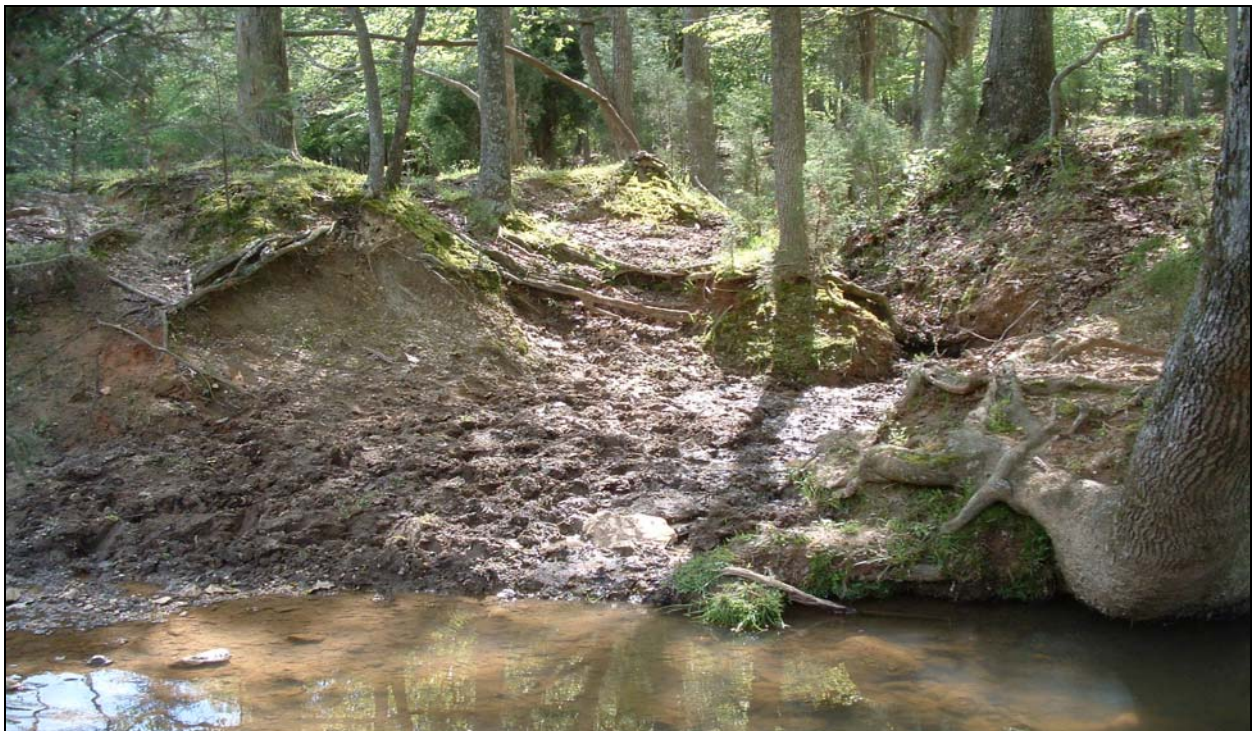
Photograph 24 – Confluence of UT3 with UTBC along right bank, significant erosion due to cattle access.
