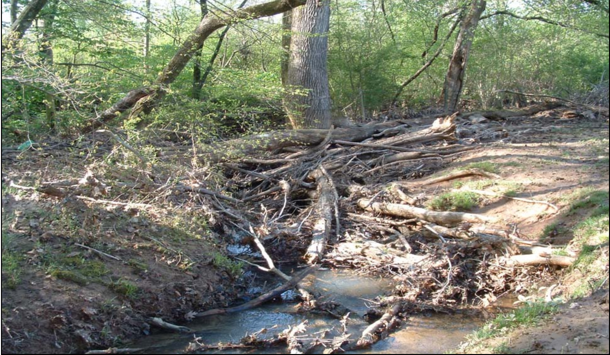
Photograph 39 – Debris jam at downstream end of project, caused by barbed wire fence crossing stream at the property boundary.
