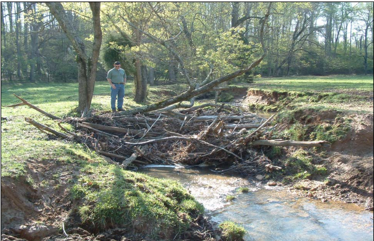
Photograph 28 – View downstream of fallen tree and large debris jam across UTBC.
