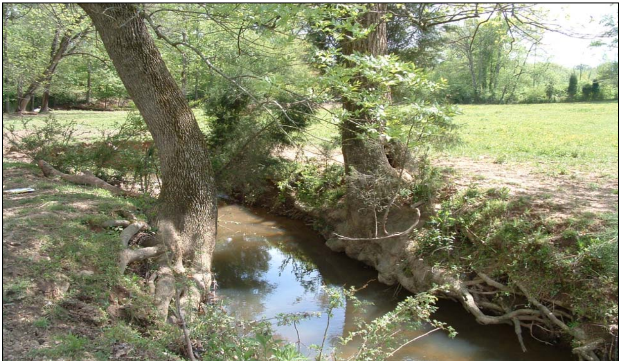
Photograph 30 – View downstream of channel constricted between large trees on each bank. Bank undercutting has left roots exposed.
