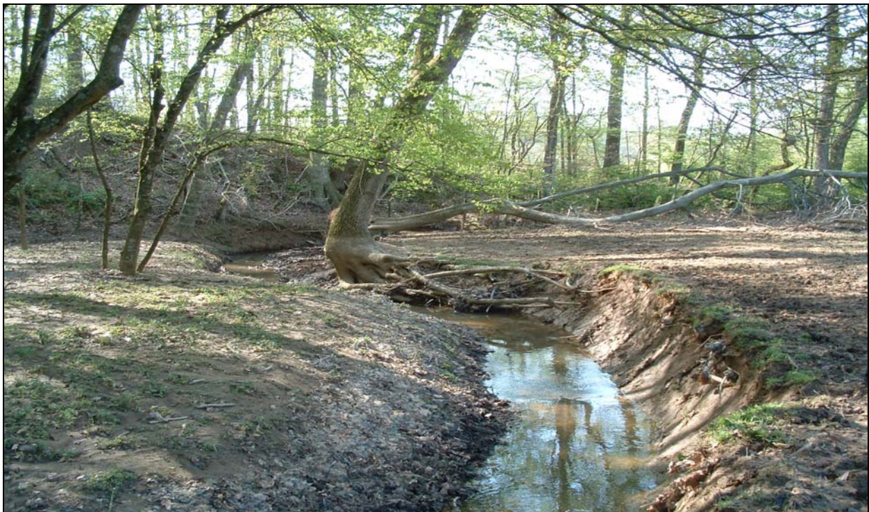
Photograph 38 – Downstream view of UTBC. Unstable banks, undercutting around large tree on right bank has left roots exposed. Further downstream, a large uprooted tree on the right bank has fallen away from stream into riparian area.
