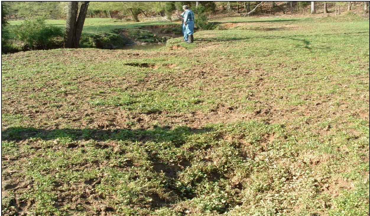
Photograph 20 – Sinkholes in right bank extending approximately 30 feet from top of bank, possibly associated with drainage tile (Station ~21+00).
