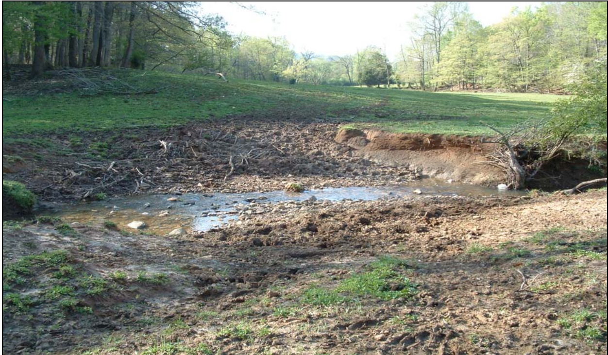
Photograph 18 – Cattle crossing at near Station 20+50. Cobbles and boulders in stream channel, possibly placed to help stabilize crossing. Banks flattened from cattle access, increasing channel width/depth ratio.
