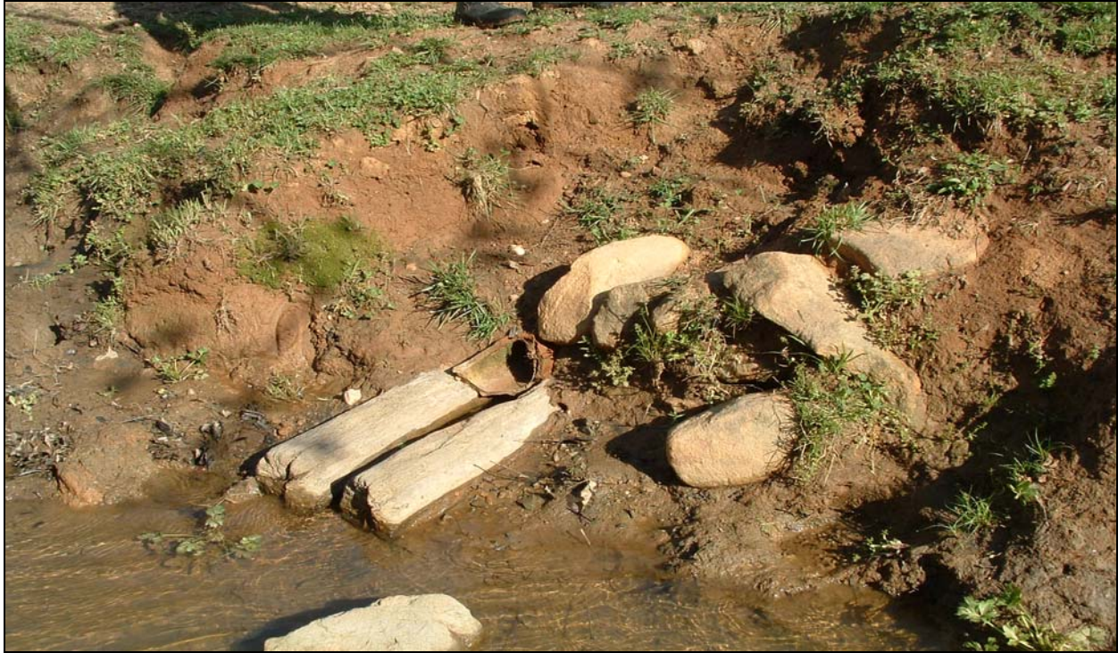
Photograph 19 – Ceramic drainage tile about four inches in diameter at base of right bank (Station ~21+00).
