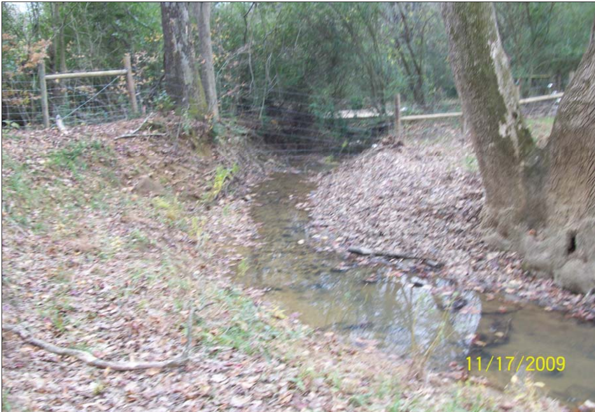
Photo Point 10d: View looking downstream towards the end of the project. 11/17/09 – MY-01
