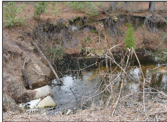
Photo 2: Pond Drainage Outlet – Concrete culverts located at the northern outfall channel and adjacent eroded soil.
