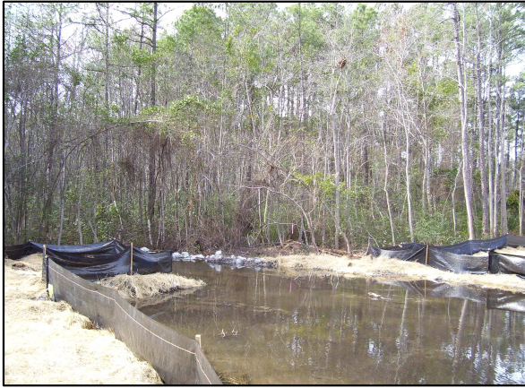
Photo 10: Temporary silt fence, spread hay, and rip-rap located adjacent to new stream channel.
