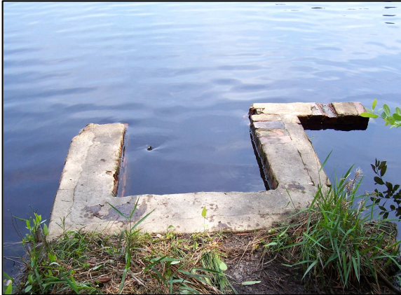
Photo 3: Pond Drainage Inlet – Brick flash board riser leading to gate valve structures located near the center of the dam.
