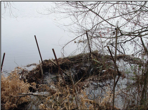
Photo 1: Pond Drainage Inlet – Brick and mortar riser structure at the northern outfall channel located within the pond at the northern extent of the dam.
