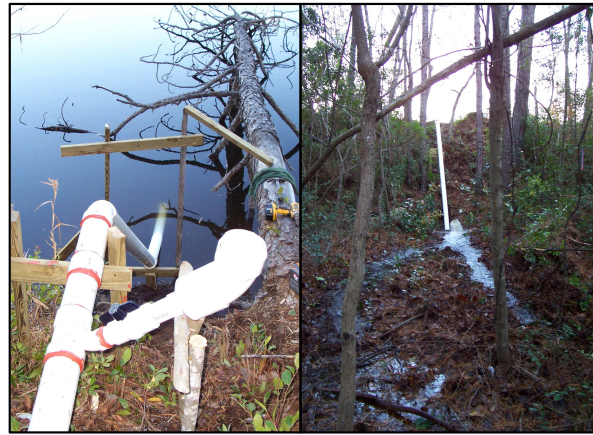
Photo 8: 4 inch siphon system installed to assist with the control of pond pool elevation following storm events.
