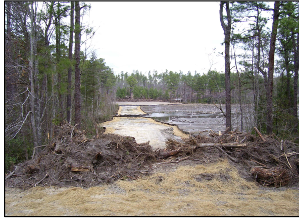
Photo 11: View of former dam from south-side looking north at erosion control measures including logging debris, silt fence, and hay bales.
