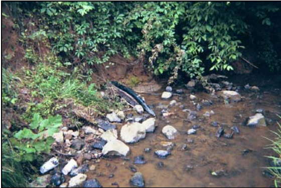
Photo 1. Exposed ABS conduit near the upstream project limits.
