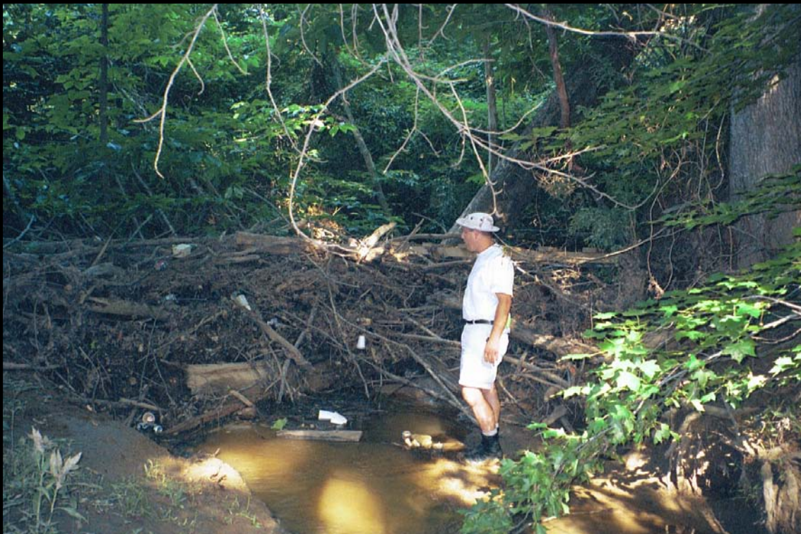
Photo 6: Large debris jam, near station 38+00, disrupts flow in McIntyre Creek at this location.
