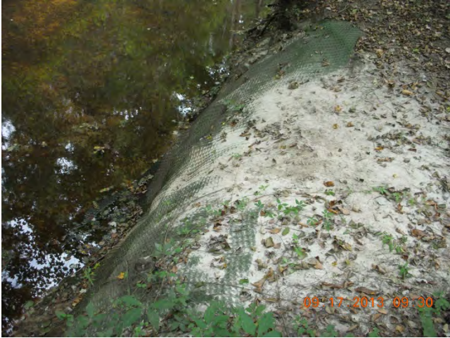
Photo 7. Sediment at berm cut
