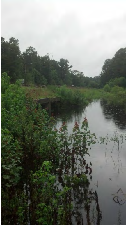
Photo 990. Canal above bankful at culvert on West Carthage Road
