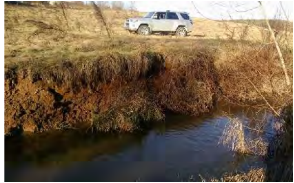
Vertical bank in the middle of R3. Channel incision and toe scour are visible.
