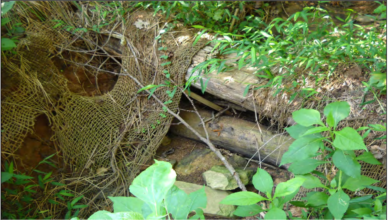
SP3: Compromised log sill structure on UT5 Taken: 8-4-2010
