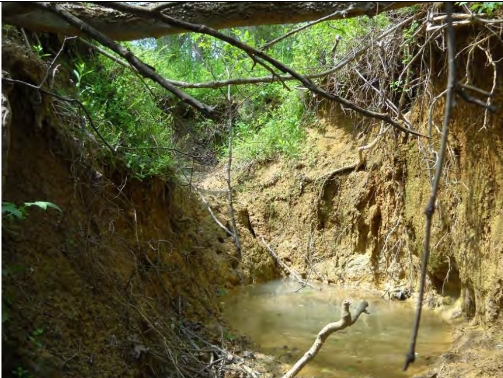
SP4: 2 foot headcut on upper UT5 (stable) Taken: 4-19-2011
