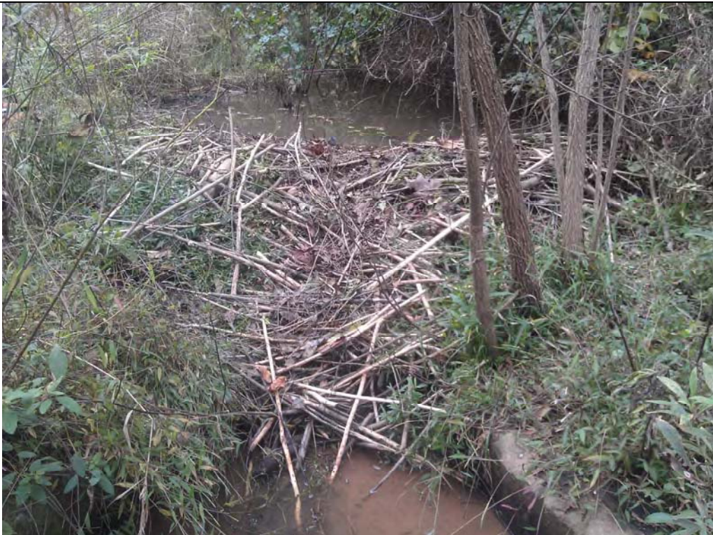
SP6: Beaver dam on lower M1 (STA 32+105) Taken: 10-18-2012
