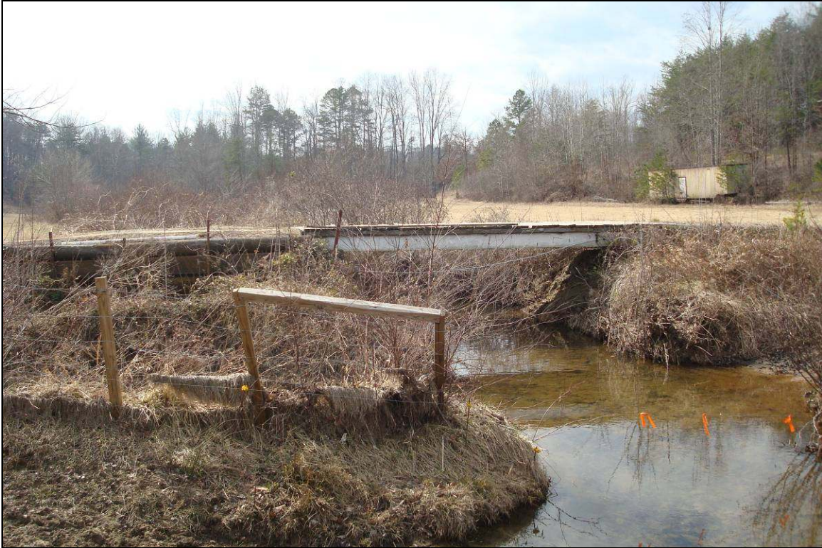
Downstream of Bridge on South Muddy Creek @ Sta 105+25 facing upstream 2/18/11 Photo No. 4
