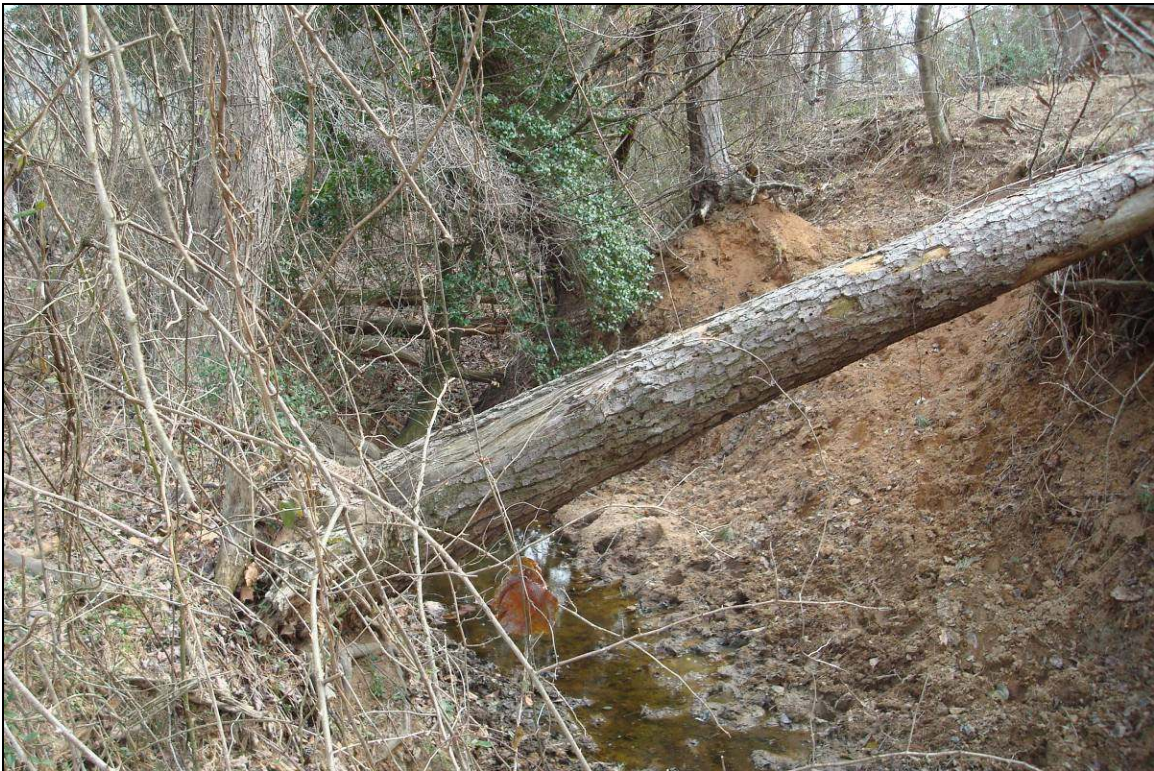
High banks and erosion on Iva Branch @ Sta 303+75 facing upstream
