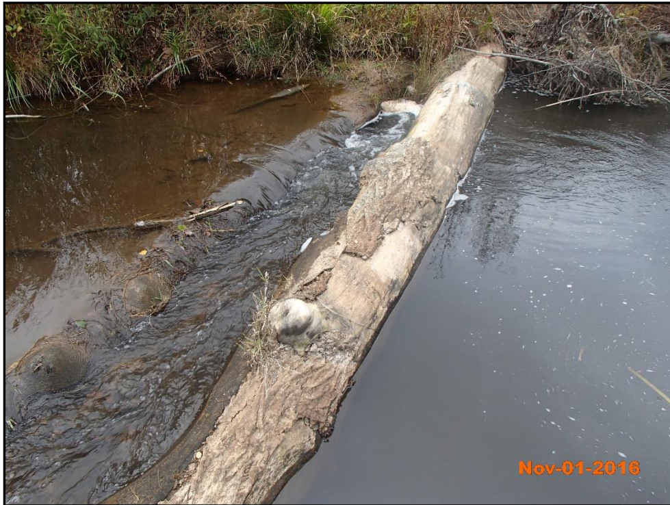
Stressed Structure – South Muddy Creek STA 108+83
