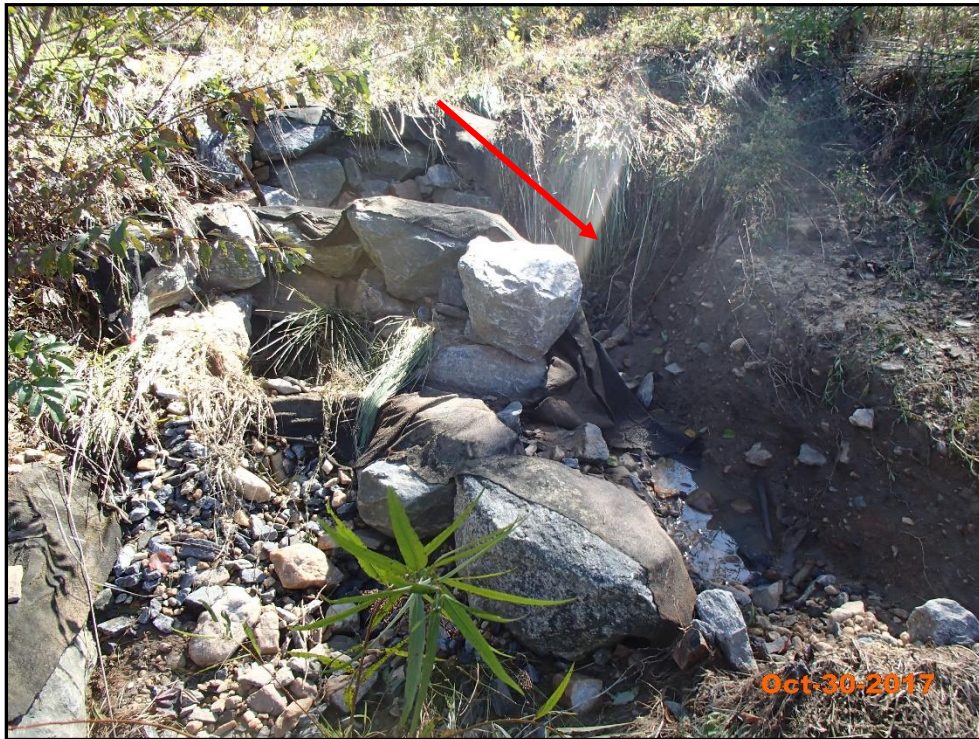
Failed Structure – Iva Branch STA 303+67 (looking upstream)
