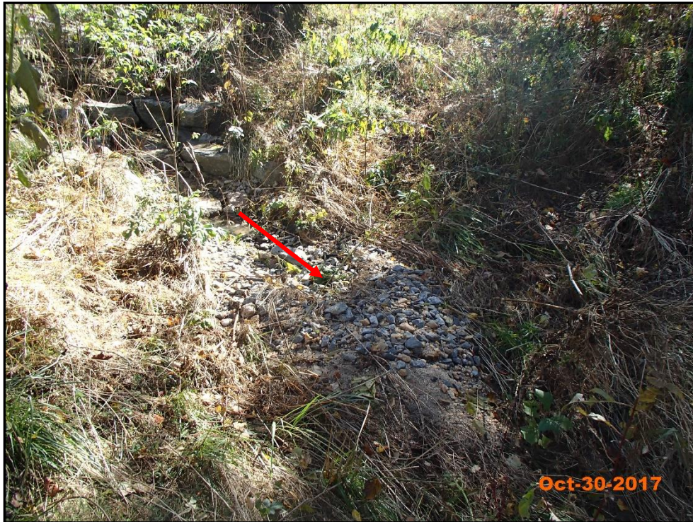
Aggradation – Iva Branch STA 302+25
