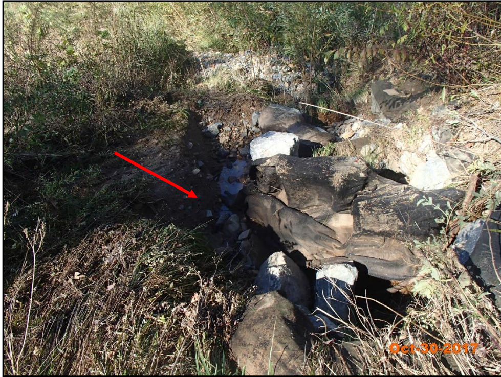
Failed Structure – Iva Branch STA 303+67 (looking downstream)
