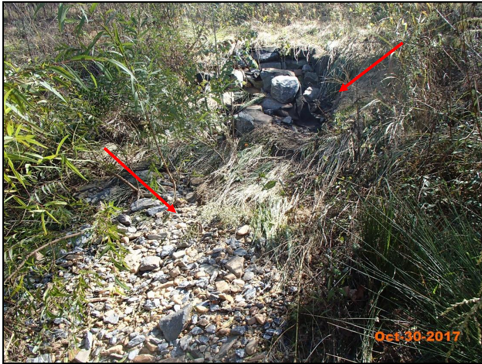
Aggradation/ Failed Structure – Iva Branch STA 303+75
