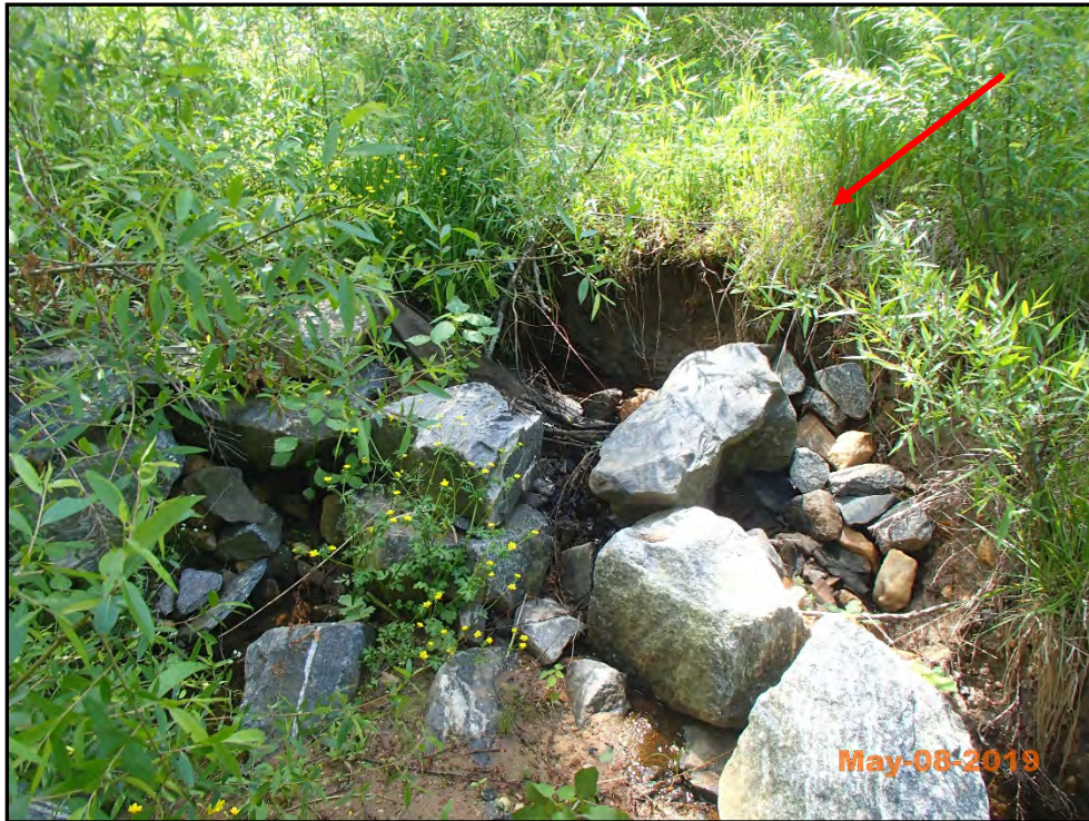
Failed Structure – Iva Branch STA 303+67 (looking upstream)
