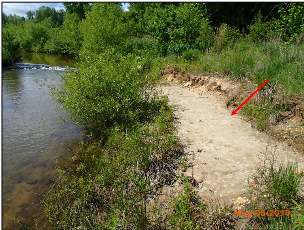
Bank Scour LDB– South Muddy Creek 109+00 (looking upstream)
