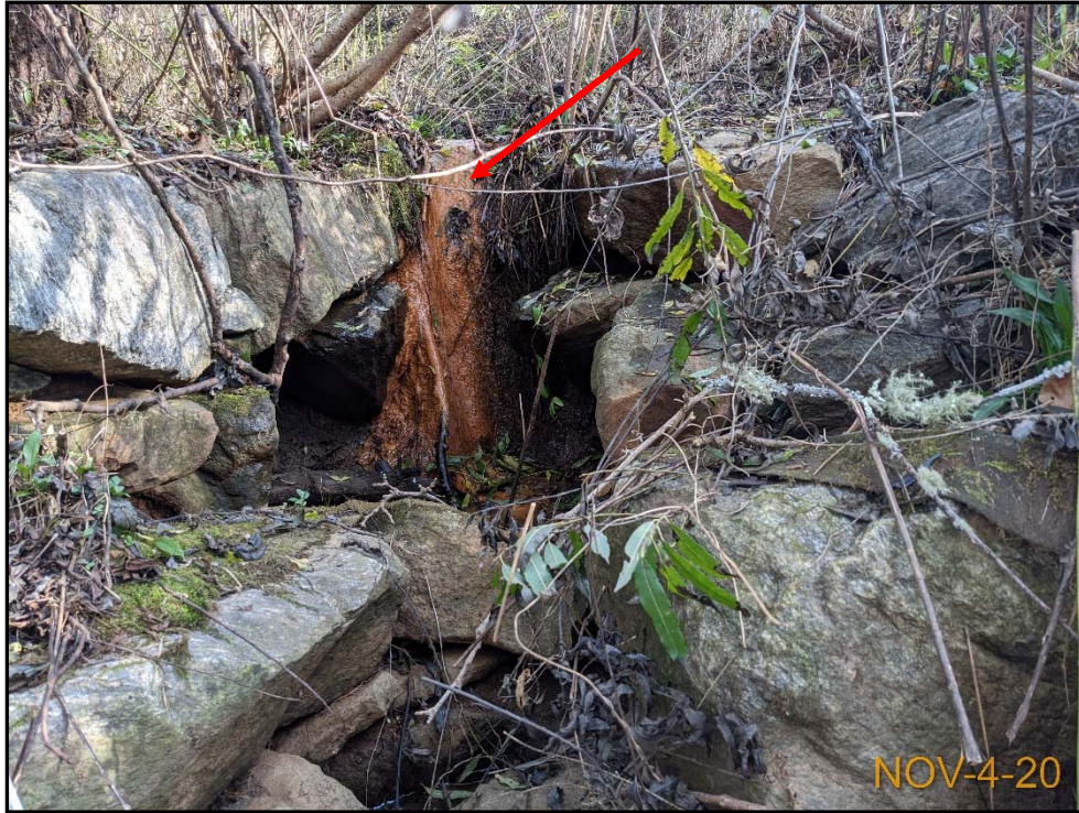
Failed Structure – Iva Branch STA 303+67 (looking upstream)
