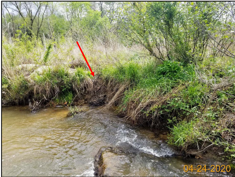
Bank Scour RDB– South Muddy Creek 109+00 (looking downstream)
