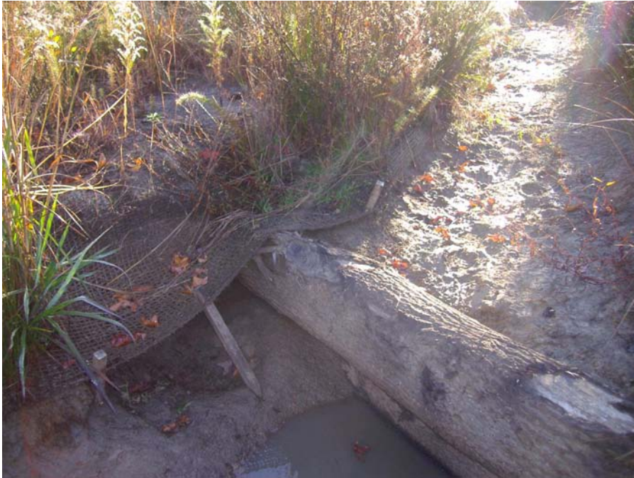
SP 1. Example of scour (STA 12+63)
