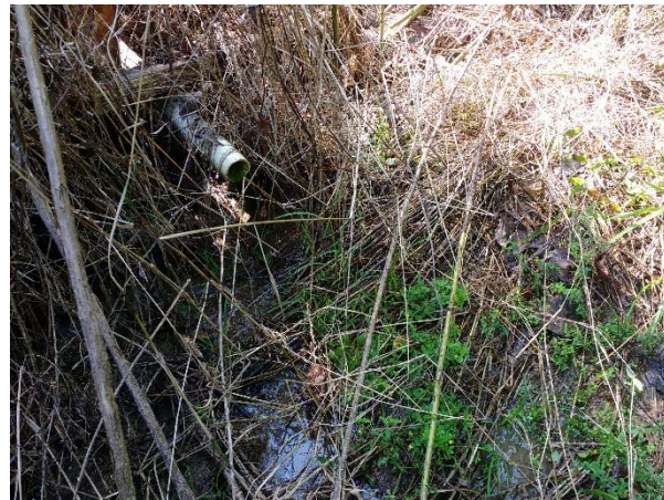
Photo 9: Outlet of T5A from a seep.
