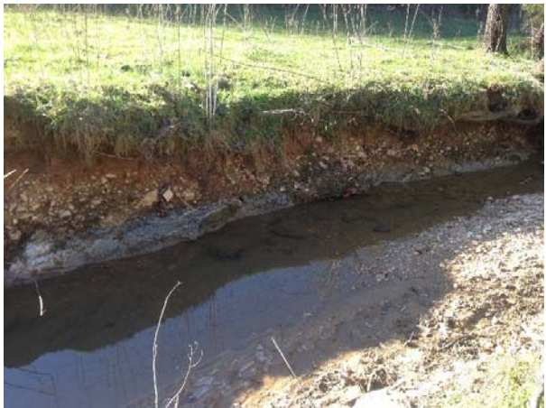
Photo 20: Active erosion on UTHC-3
