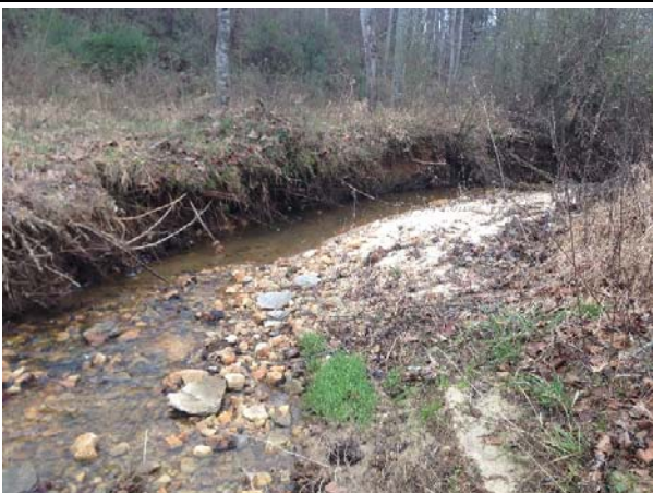
Photo 23: Active erosion on UTHC-4
