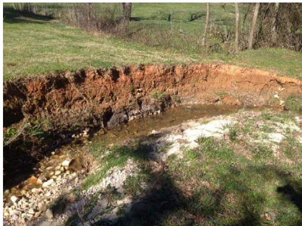
Photo 3: Active erosion on UTHC-1 just upstream of confluence with T1
