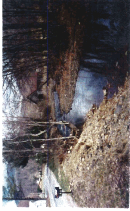
Looking upstream from station 5+31. This area will have structures installed to confine the thalweg towards the center to prevent any further bank erosion and to protect the road shoulder.
