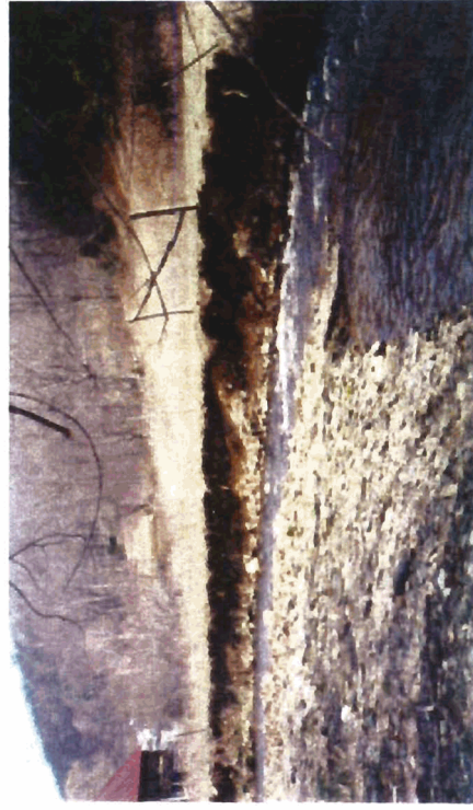
Major bank erosion site, approximately 110' in length at station 3+33.
