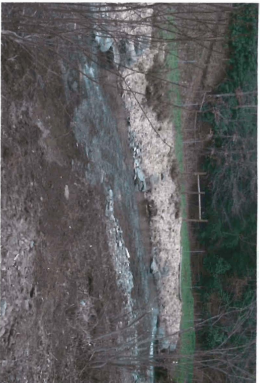
Bank after repairs using three rock vanes, one rock weir, and bank reshaping, November 2004.
