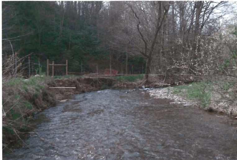
After November 19, 2003 flood. Notice that 6 ft of the watering tank drainage pipe is exposed.
