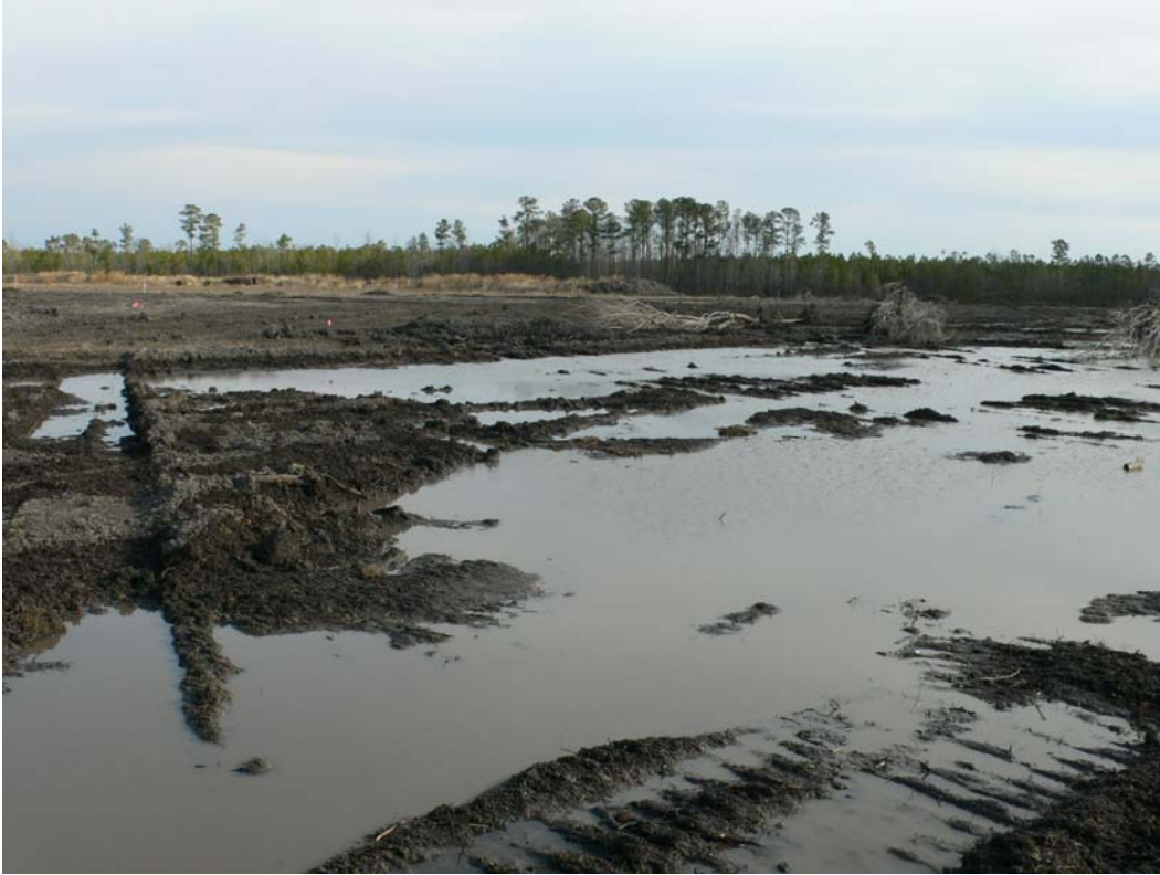
Photo 5. Widespread inundation occurring during construction.
