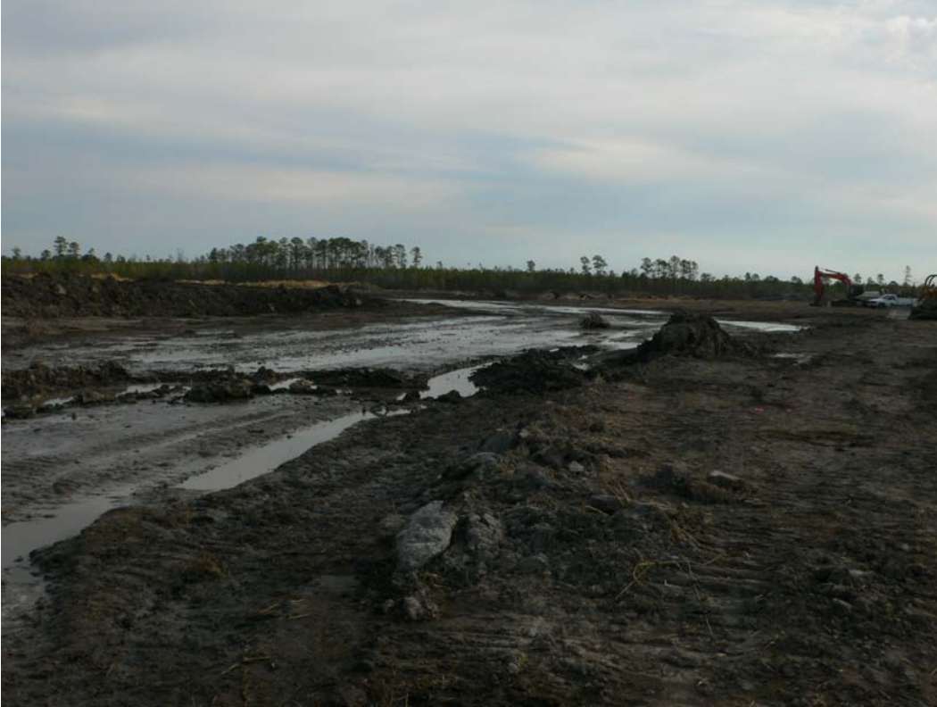
Photo 4. Wet conditions encountered during construction.
