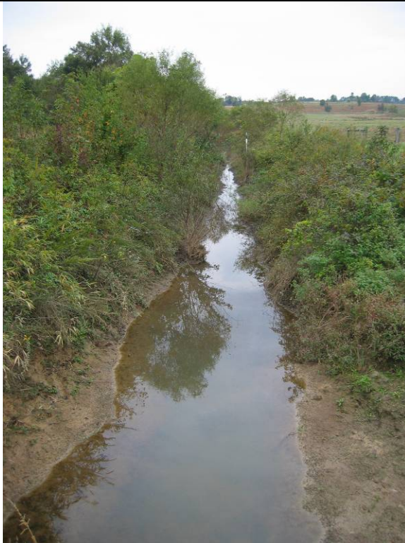
Photo 10: Lateral ditch at southern end of site flowing to Swift Creek (10/18/04 – Typical)
