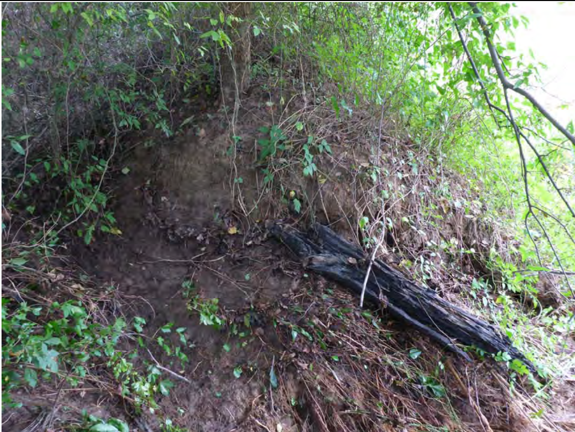
WP6 (September 10, 2014) Cross-sectional view of southern breach in berm from Swift Creek.. Photo is facing south.
