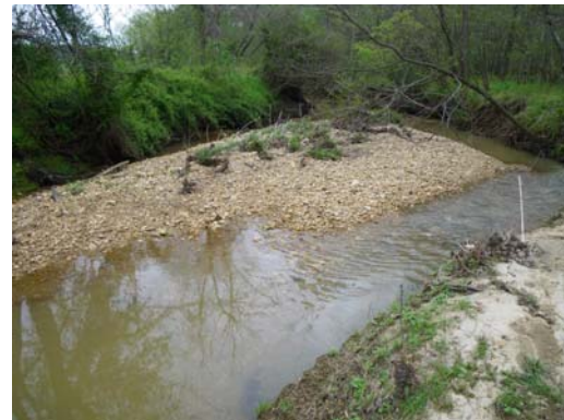
Moores Fork, looking downstream from station 42+00; mid-channel deposition, bank erosion; April 20, 2011
