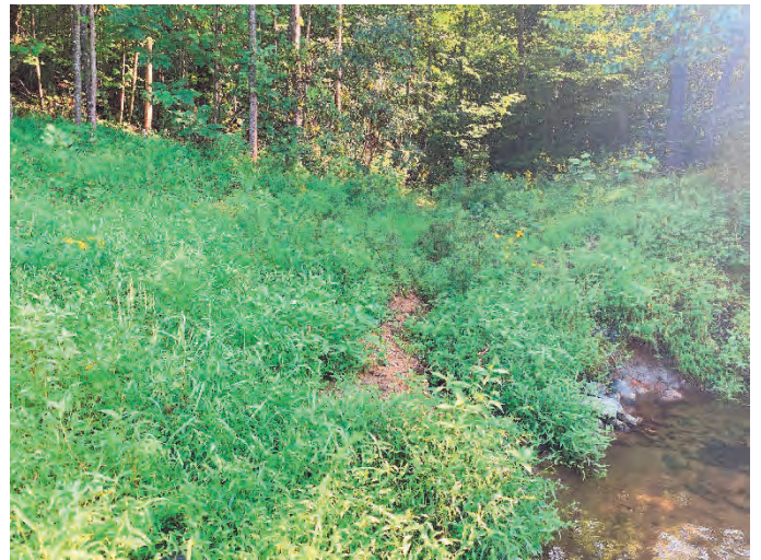
UT8/Wetland outlet repair at confluence with Moore's Fork – 9/7/2021
