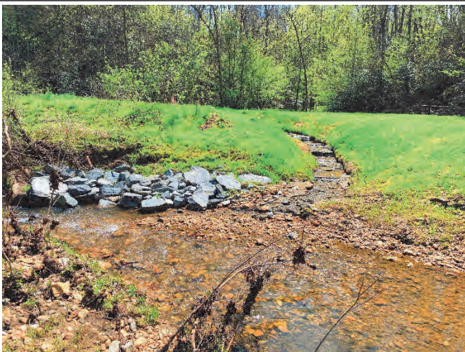
UT10/Wetland outlet repair at confluence with Moore's Fork – 4/19/2021
