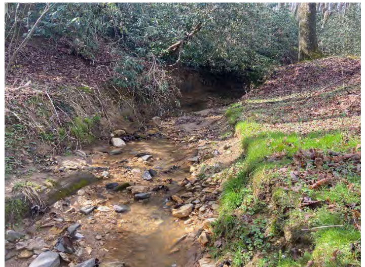
PP48 – Silage Reach 2, looking upstream (04/06/2022)
