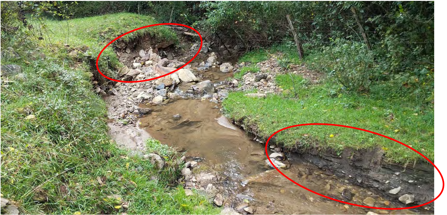
Formerly stable banks, now both are actively eroding after storm event requiring bank grading, stabilization, and bench grading (Area F).
