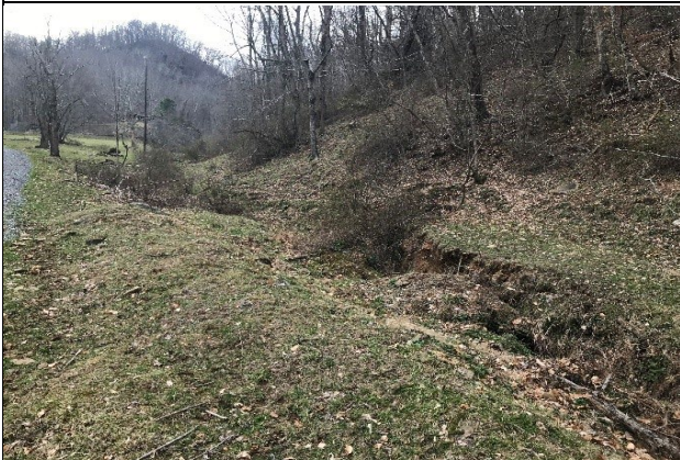
Photo 11: Erosion and instability along T9. 1/24/2018
