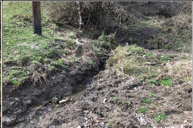
Photo 12: Headcut and erosion along T8. 1/24/2018
