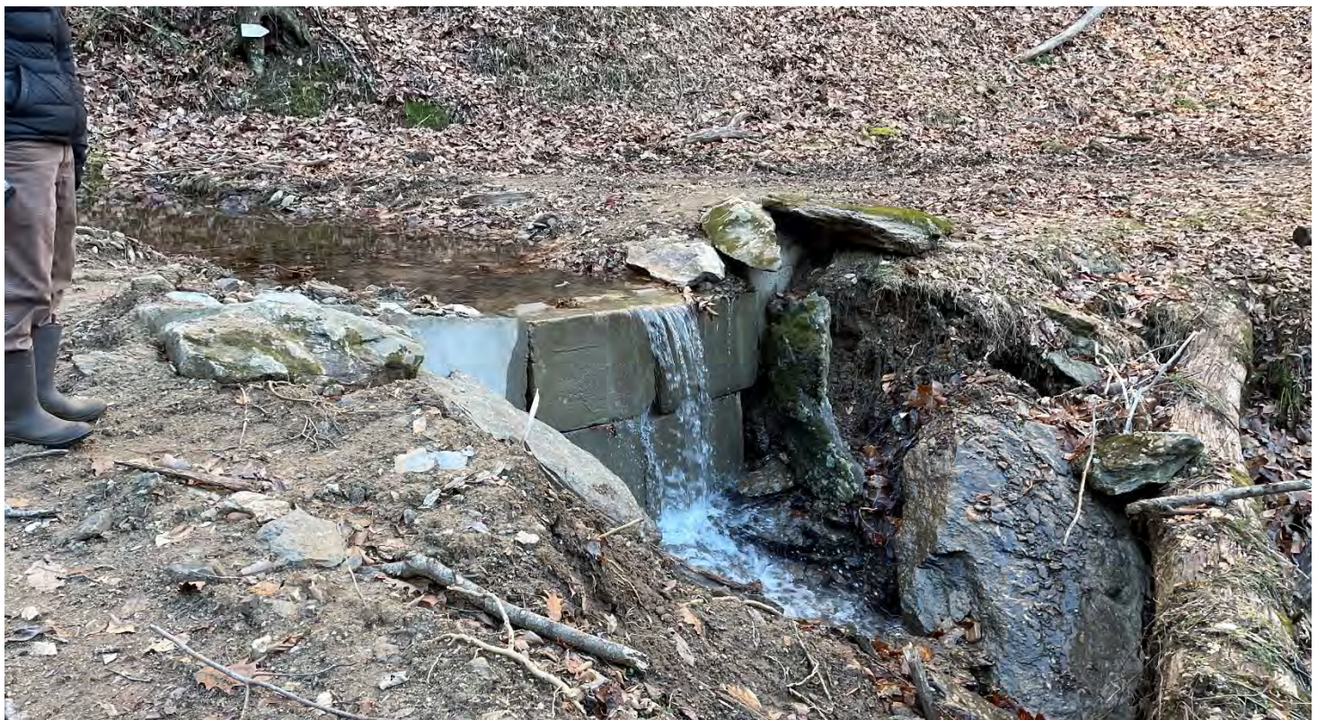
Washed-out culvert was temporary repaired by the landowner with a ford secured with concrete blocks (Area D).
