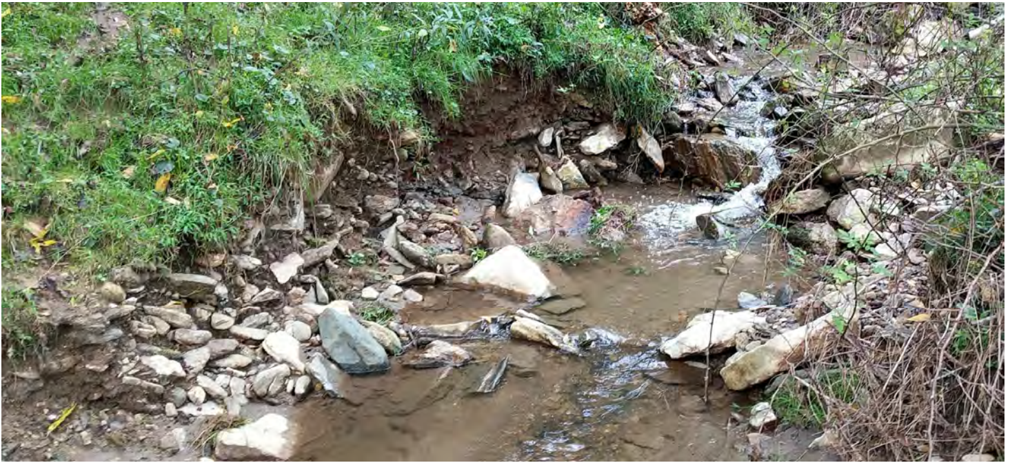
Formerly stable bank on Morgan Branch, now actively eroding after storm event, will require bank grading, stabilization, and bench grading (Area F).
