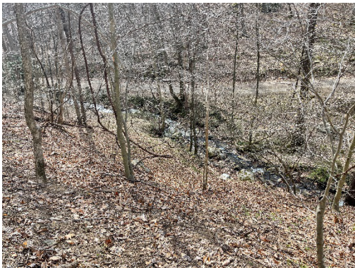
MB-2 looking downstream. There is an access road along the right bank.
