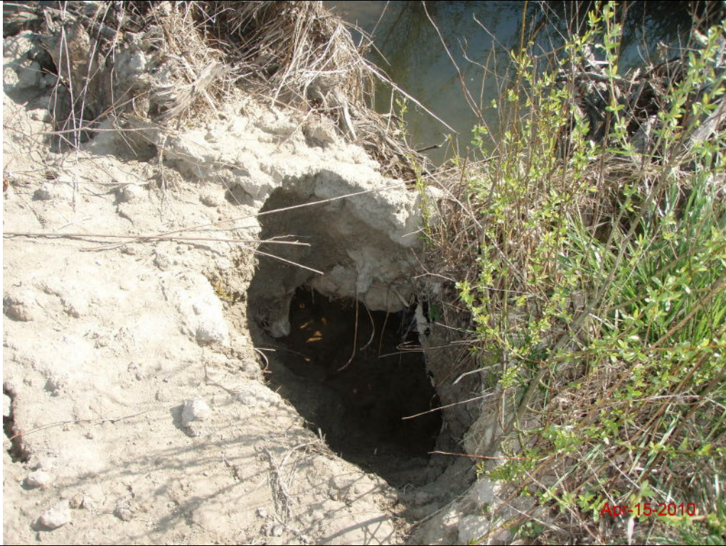
SPA13 Morgan Creek Sta. 1014+50 – Stressed Bank
