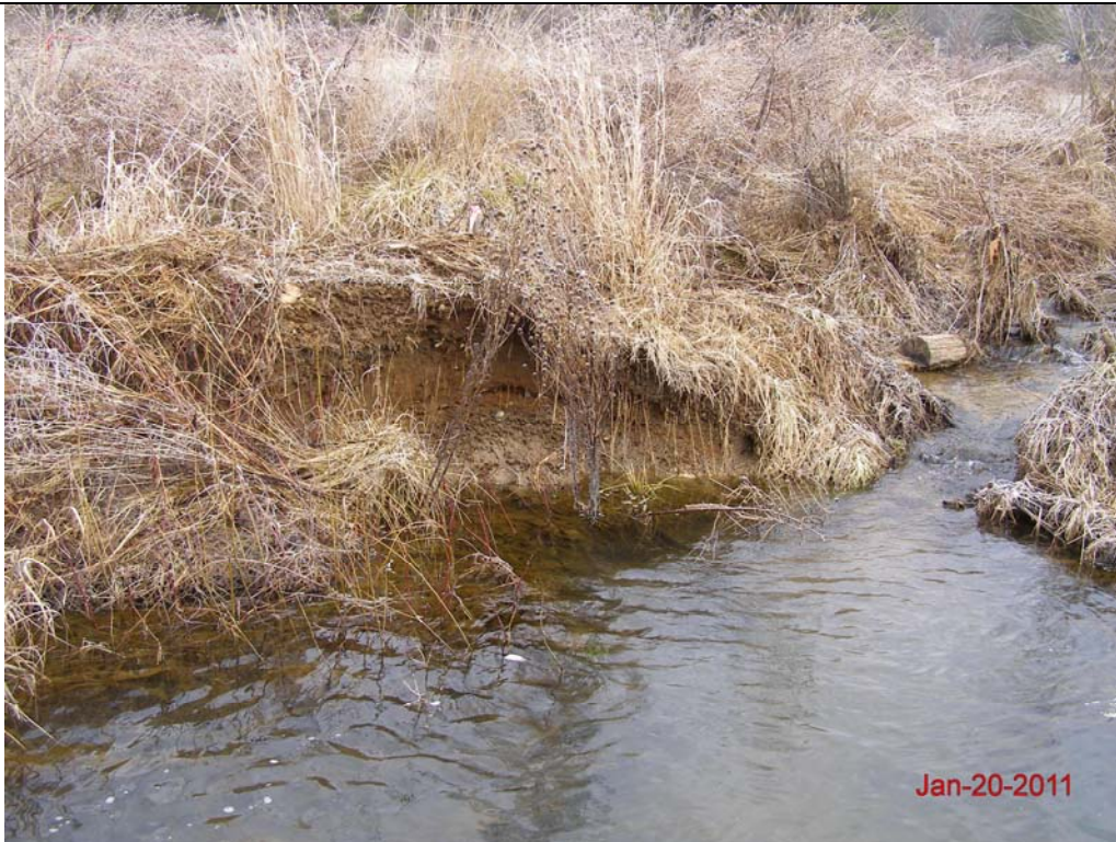
SPA 21 Morgan Creek Sta. 1029+40 – Bank erosion due to thalweg not centering
