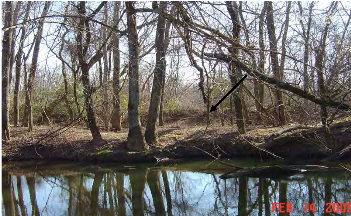
Photo 8: Existing Southern Berm as viewed from the Northern bank of Morgan Creek
