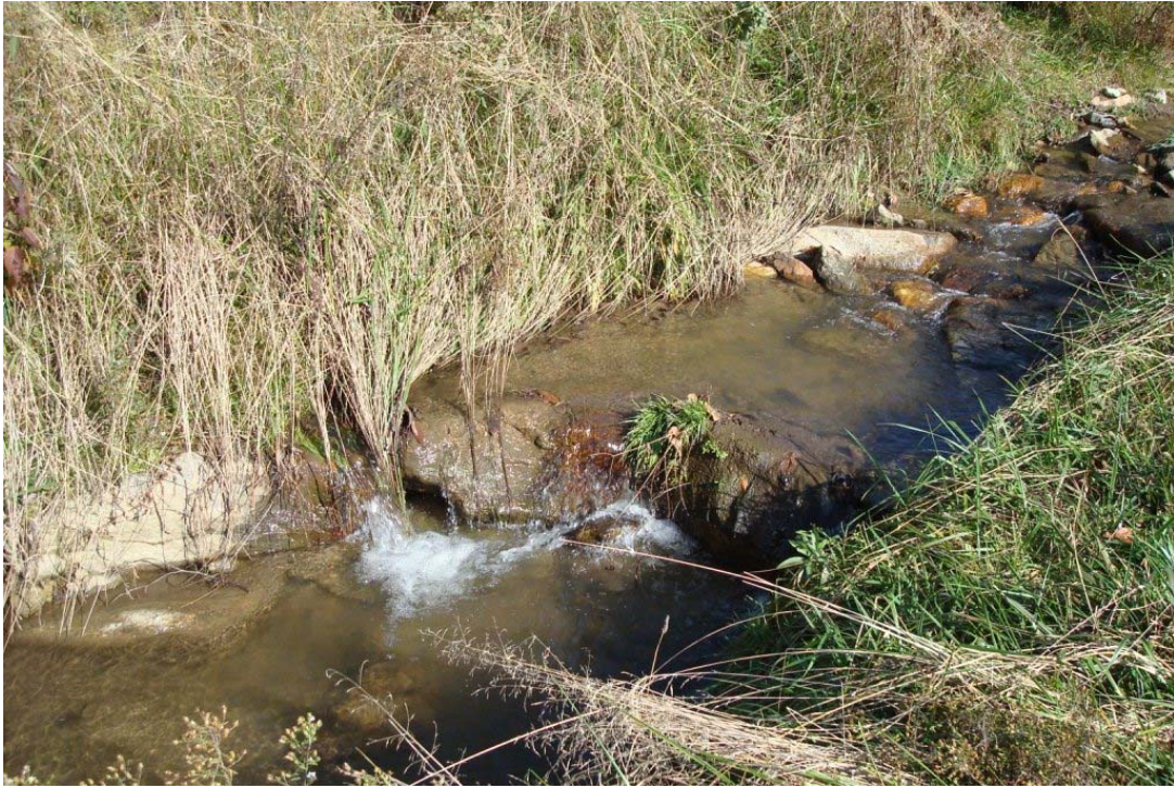
Excessive Drop on Boulder Run Arch, Morgan Cr, Sta 102+47 (Appears to be holding) Year 1 10/30/09 Photo No. 3
