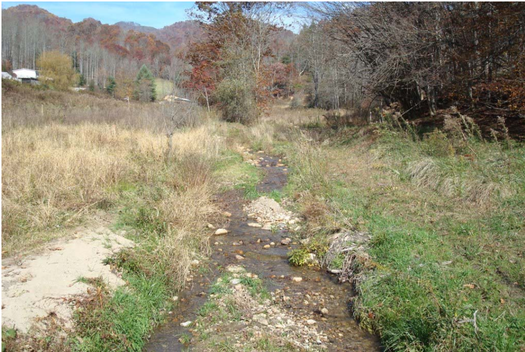
Deposition caused by pipe blockage, Morgan Cr, Sta 118+05
