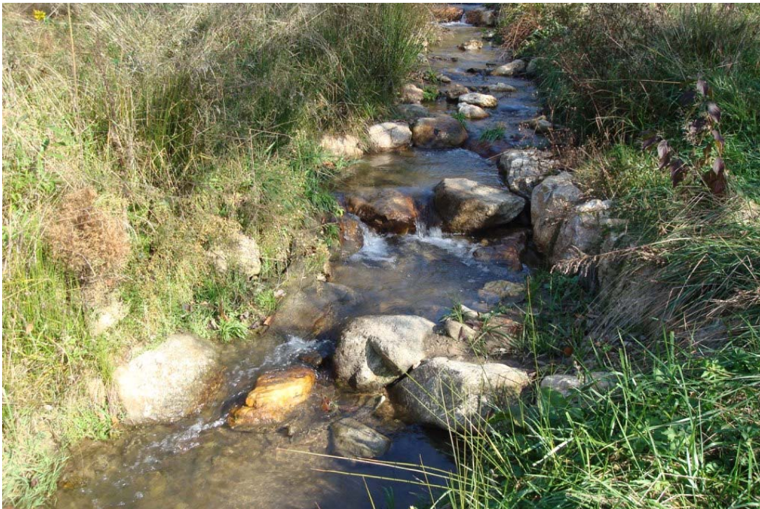
Gap in Structure Baffle, Morgan Cr, Sta 102+06 (Appears Stable)
