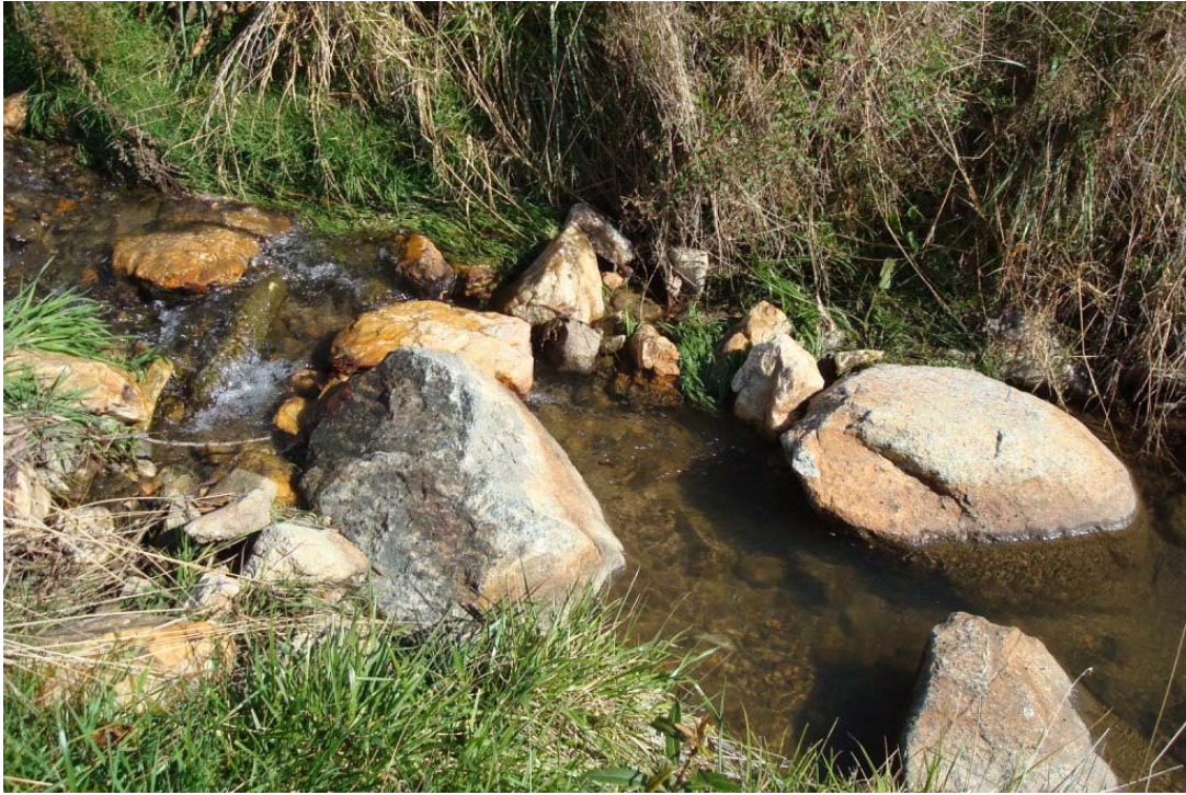
Material scoured out of Boulder Run Structure, Morgan Cr, Sta 112+30 (Grade is being held by upper portion of structure)
