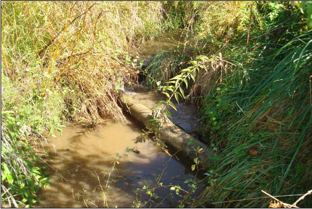
Minor piping of log hook, Morgan Cr, Sta 102+90
