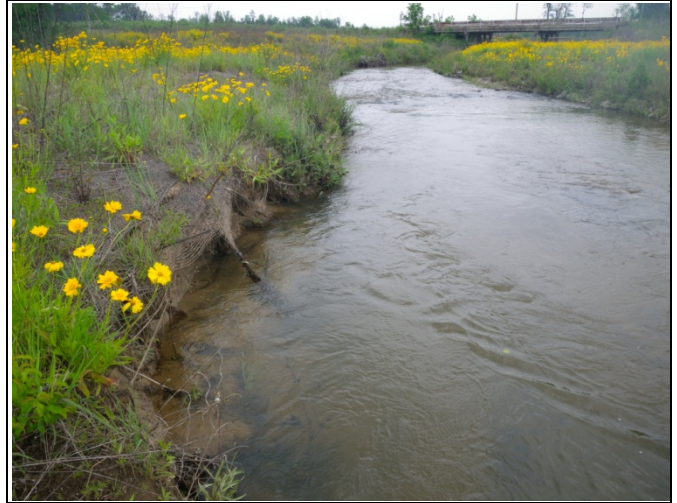
SPA2 – Localized scour along left bank from eddying within the riffle (looking downstream)
