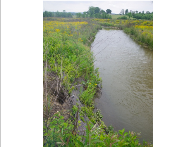
SPA1 – Right bank separating/overhanging from poor compaction and scour along toe of bank (looking upstream)
