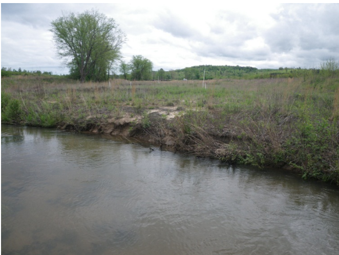
SPA2-3 – Localized scour along right bank within a riffle from the lack of thalweg centering downstream of a meander bend (looking downstream from left to right bank)
