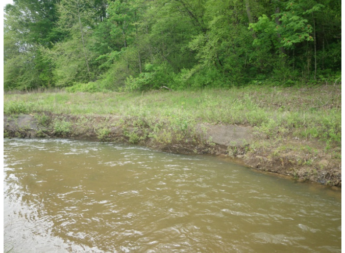
SPA2-2 – Right bank/brush mattress separating from poor compaction and scour along toe of bank (looking downstream from left bank to right bank)
