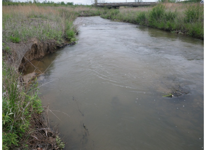
SPA1-2 – Localized scour along left bank from eddying within the riffle (looking downstream)
