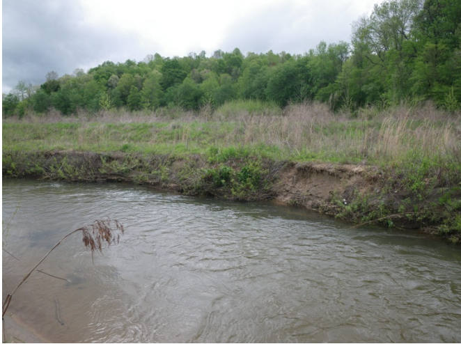
SPA1-1 – Right bank/brush mattress separating from poor compaction and scour along toe of bank (looking downstream from left bank to right bank)
