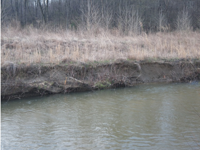
SPA1-1 – Right bank/brush mattress separating from poor compaction and scour along toe of bank (looking upstream from left bank to right bank)
