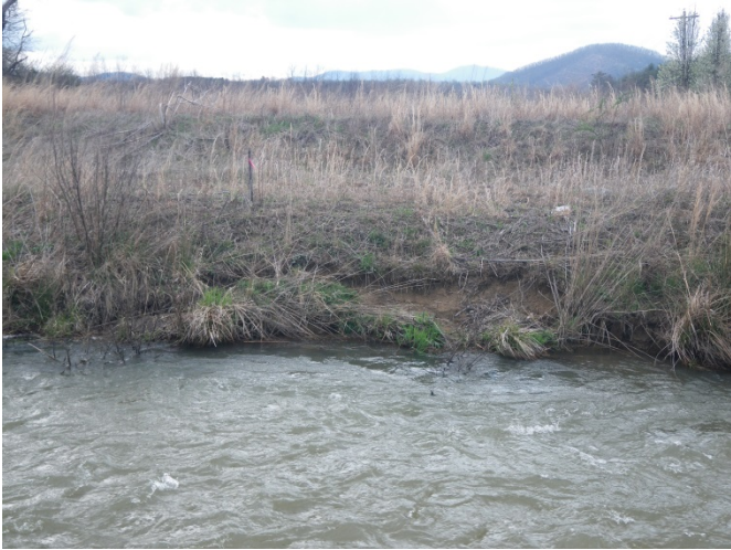
SPA3-2 – Localized scour along right bank downstream of Sain Rd. Bridge. Result of high shear stress caused by steep riffle (looking across from left to right bank)
