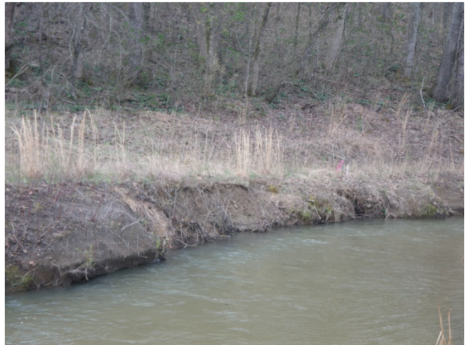
SPA2-2 – Right bank/brush mattress separating from poor compaction and scour along toe of bank (looking upstream from left bank to right bank)
