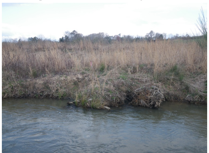
SPA3-1 – Localized scour along left bank behind rootwads (looking across from right to left bank)
