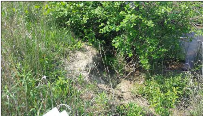
SPA4-3 – Area of right bank erosion caused by flow diversion around beaverdam.
