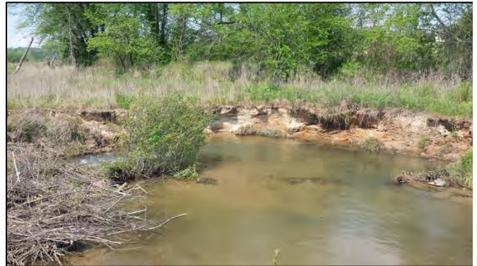
SPA4-4 – Large area of left bank erosion caused by flow diversion around beaverdam.
