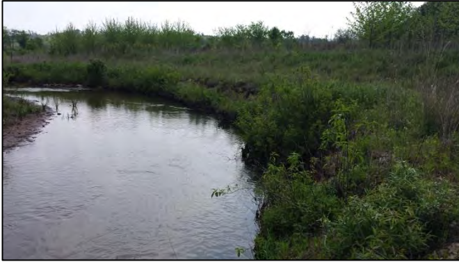
SPA1-1 – Right bank/brush mattress separating from poor compaction and scour along toe of bank (looking downstream). Appears to be stabilizing with vegetation.
