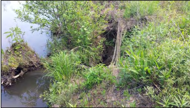
SPA4-1 – Localized scour along right bank behind rootwads (looking downstream from right bank)
