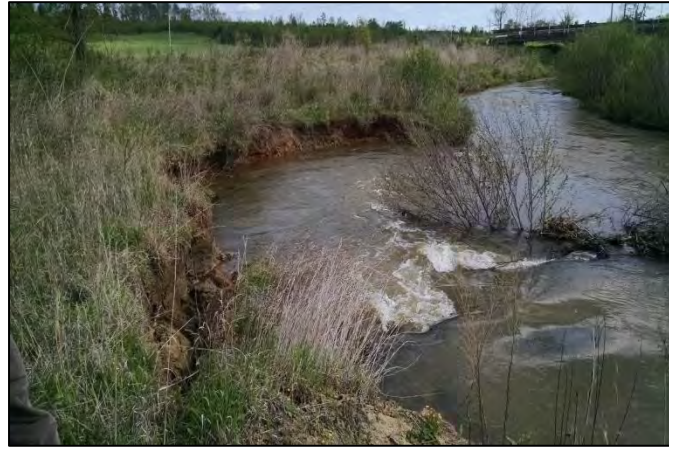
Area of bank erosion prior to implementation of maintenance work in November 2015.
