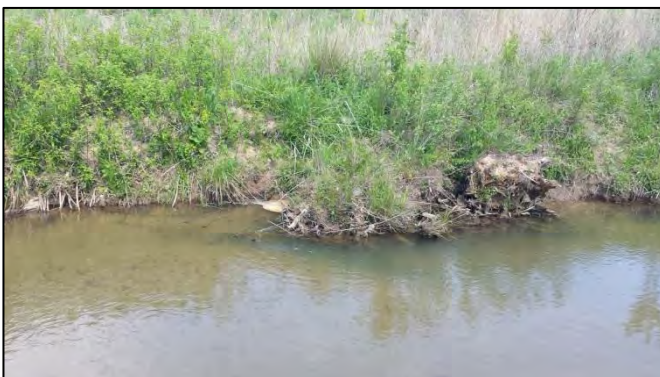
SPA3-1 – Localized scour along left bank behind rootwads (looking across from right to left bank)
