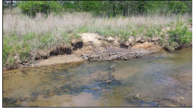
SPA1-2 – Localized scour along left bank from eddying within the riffle (looking downstream)
