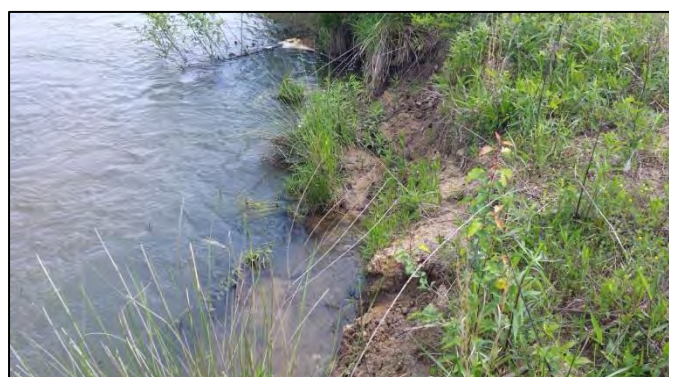
SPA3-2 – Localized scour along right bank downstream of Sain Rd. Bridge. Result of high shear stress caused by steep riffle (looking downstream from right bank)
