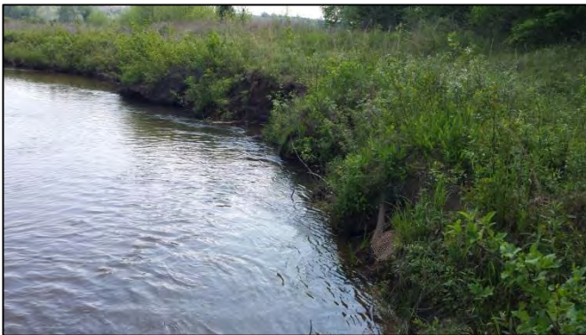
SPA2-2 – Right bank/brush mattress separating from poor compaction and scour along toe of bank (looking downstream from right bank)
