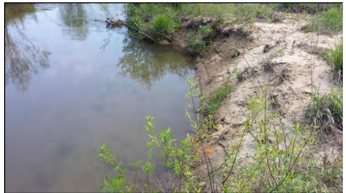
SPA2-3 – Localized scour along right bank within a riffle from the lack of thalweg centering downstream of a meander bend (looking downstream from right bank)
