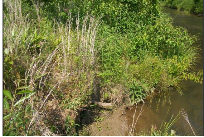
SPA 5-1 – Localized area of scour on left bank (5-25-16))
