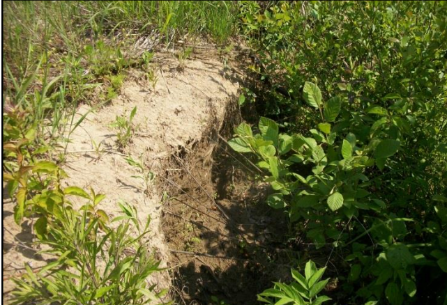
SPA4-1 – Localized scour along right bank behind rootwad and compromising the structures (5-25-16).
