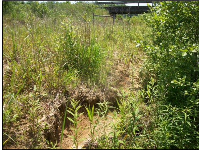
SPA 5-6 – Scour and bank slumping along right bank downstream of Sain Rd. Bridge (5-25-16).
